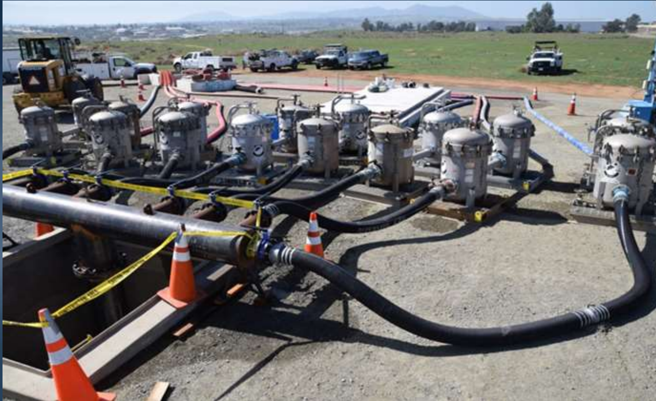
Quagga Mussel Filtration during Dewatering
