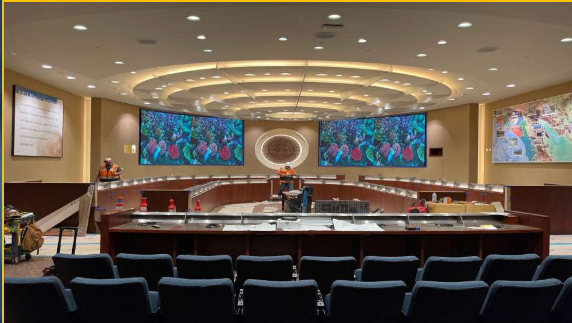
Audio visual and lighting upgrades in board room
