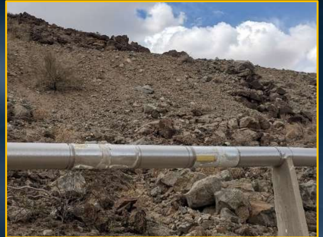
Above-ground potable water pipe
