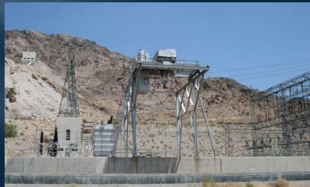
Hinds Pumping Plant
