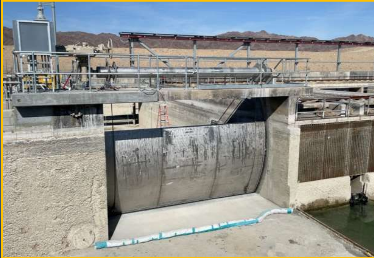
Installed Radial Gate (canal side)
