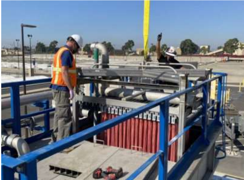
Staff removing an MBR cassette for inspection at the demonstration facility
