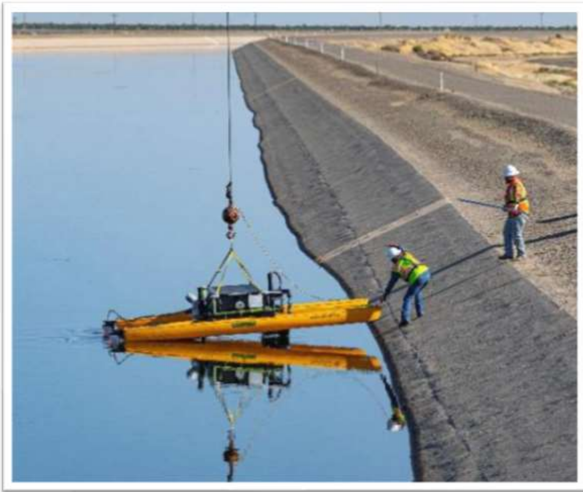
DWR staff lowers the waterborne vessel into the California Aqueduct with the help of a crane. (Credit: California Department of Water Resources)
