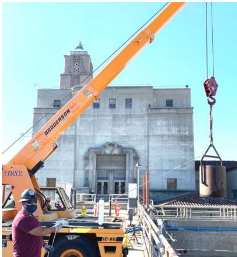
Staff using a miner's bucket to remove debris in a sedimentation basin at the Weymouth plant
