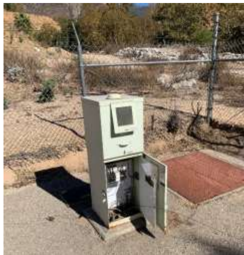
Vandalized meter cabinet along the Inland Feeder
