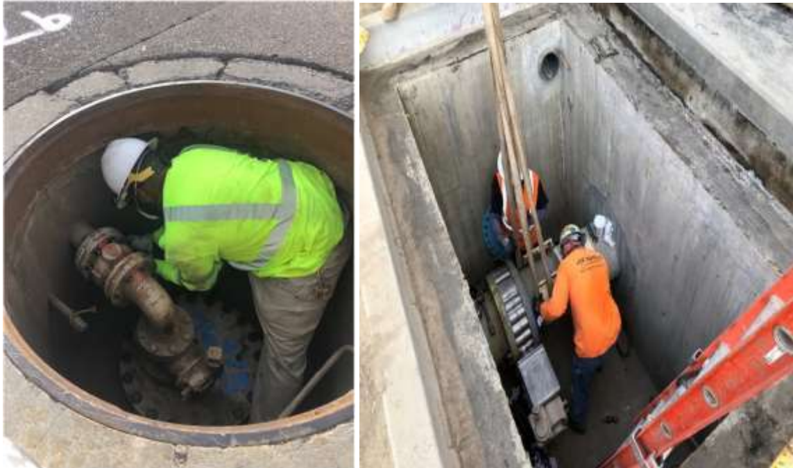
Staff installing a pipeline access flange (left) and surge valve (right) during the EVF shutdown
