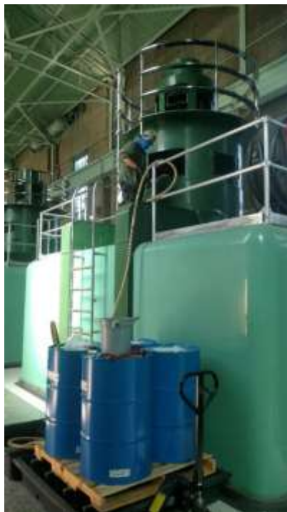
Staff changing oil in a 12,500hp motor at the Eagle Mountain pumping plant
