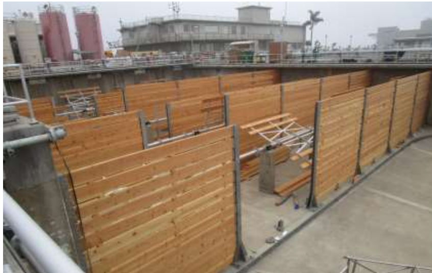
Diemer West Basin and Filter Building Rehabilitation – Installing new baffle walls and flocculators at Basin 7 (looking south-east)
