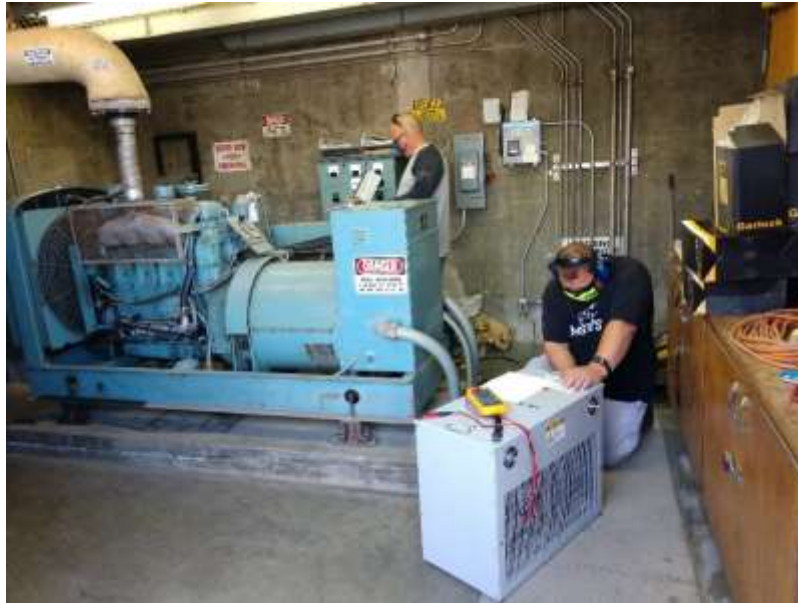
Staff testing the emergency generator at Live Oak Reservoir
