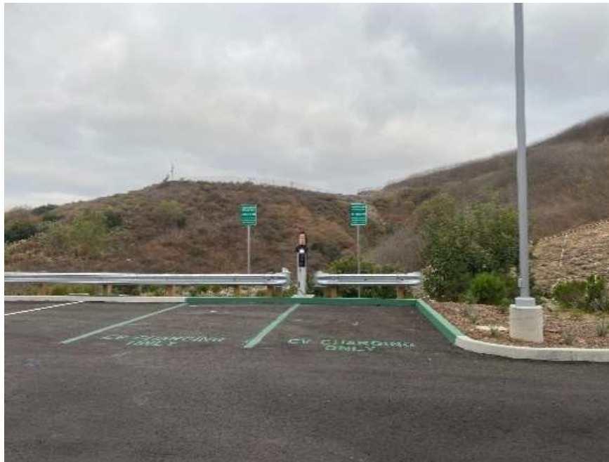
Charging station at Diemer Filtration Plant
