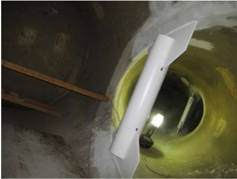
Interior view of prefabricated reinforcements at pipe joints in the Perris Pumpback facility
