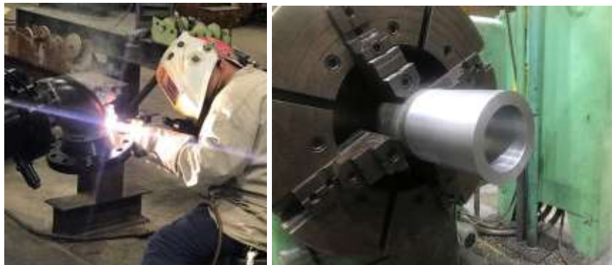
Staff welding coupling (left) and completed machining of new front cushion (right) for hydraulic actuator for DWR
