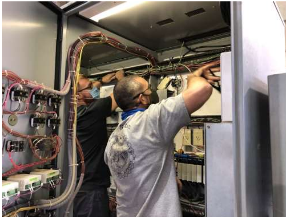
Staff installing a new PLC for solids handling at the Skinner plant
