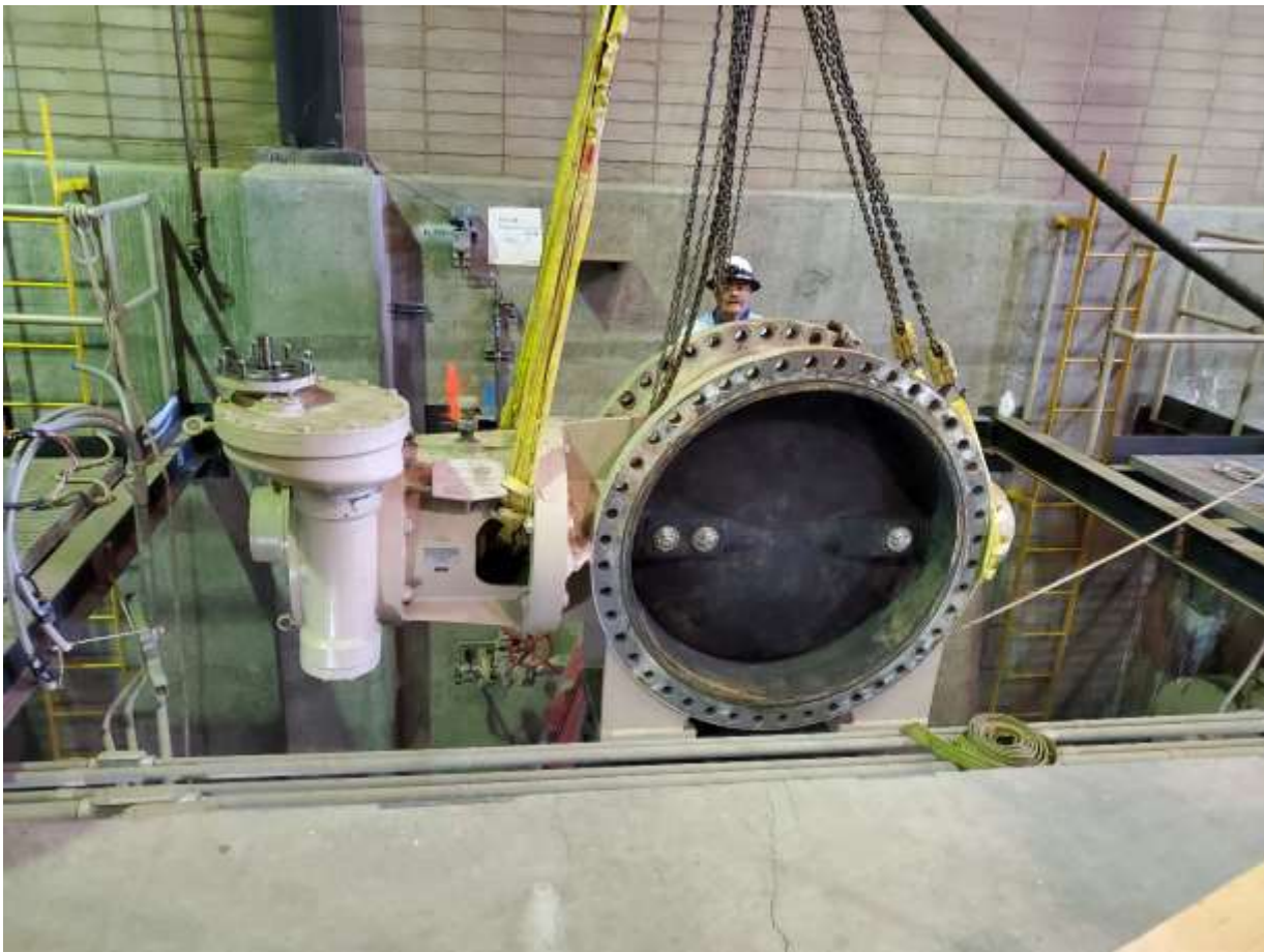
Staff removing a large valve to allow for pipe access at Perris PCS
