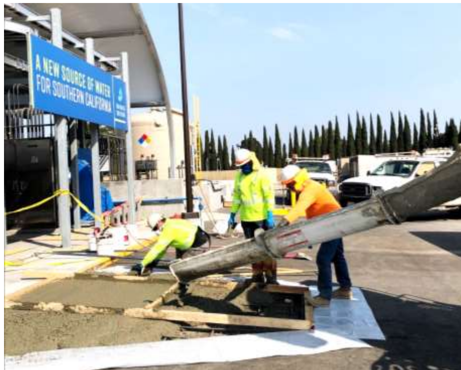
Staff pouring concrete for a new access ramp at the demonstration facility
