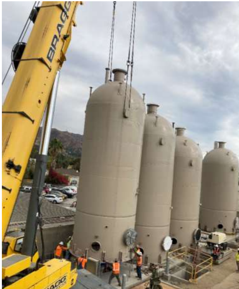
Greg Avenue Pump Station Rehabilitation—Installing (fourth) surge tank, view to the northeast
