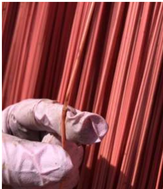
Staff inspecting a damaged membrane fiber
