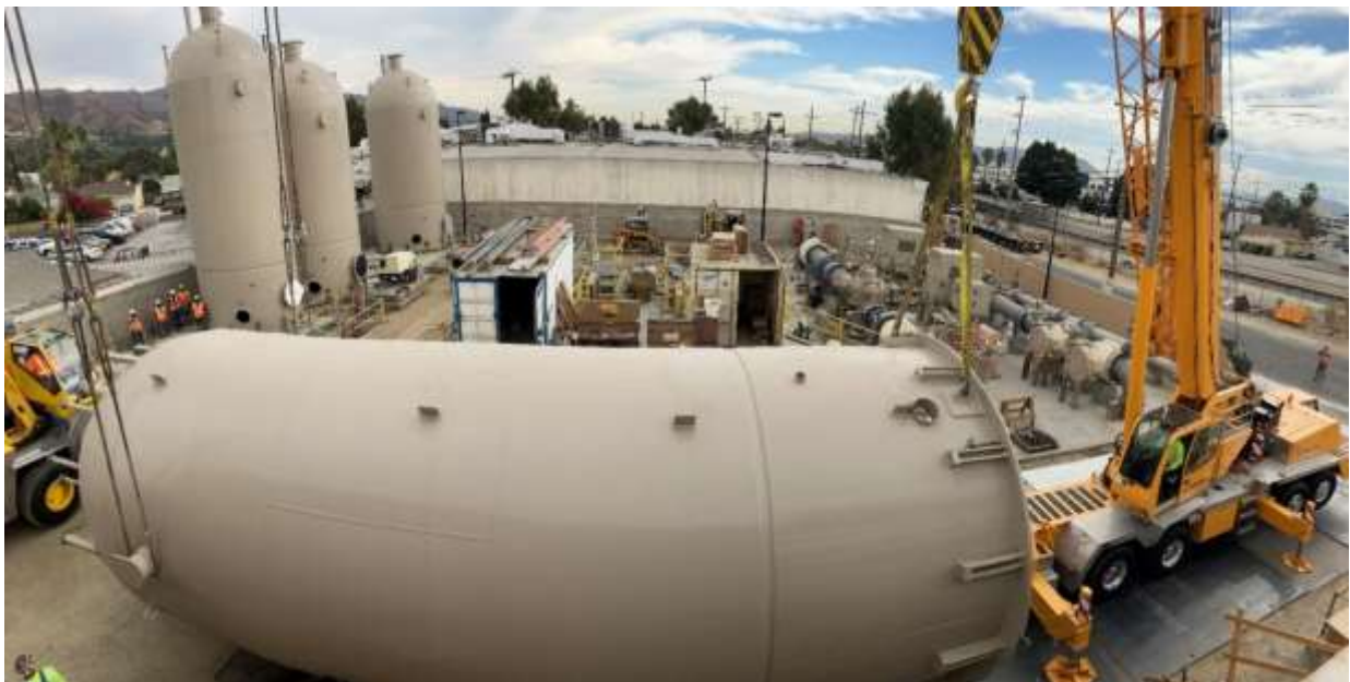
Installation of surge tanks at Greg Avenue pump station during the EVF shutdown
