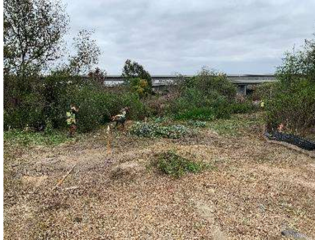
Vegetation clearing to allow access to the worksite along the Orange County Feeder
