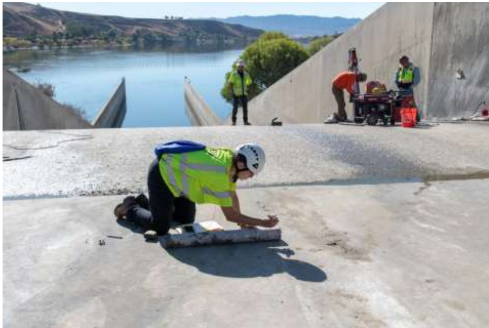
On November 6, 2019, coring work is being done on Castaic Dam's stream release chute as part of the Castaic Dam Modernization Program. (Credit: California Department of Water Resources)
