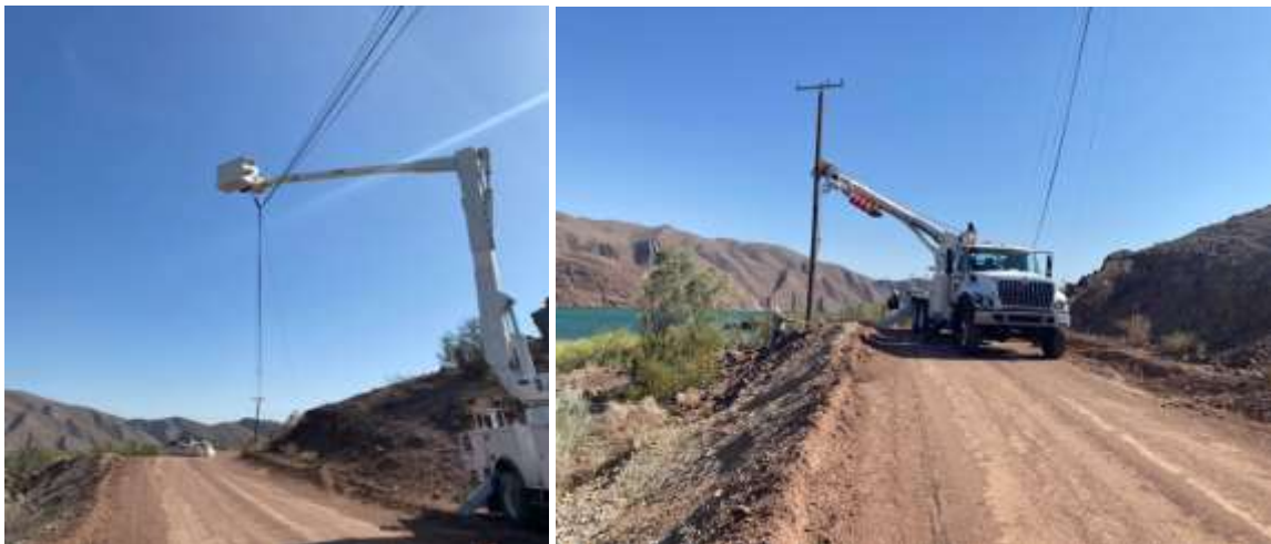
Staff replacing power pole and crossarms damaged by high winds near Copper Basin
