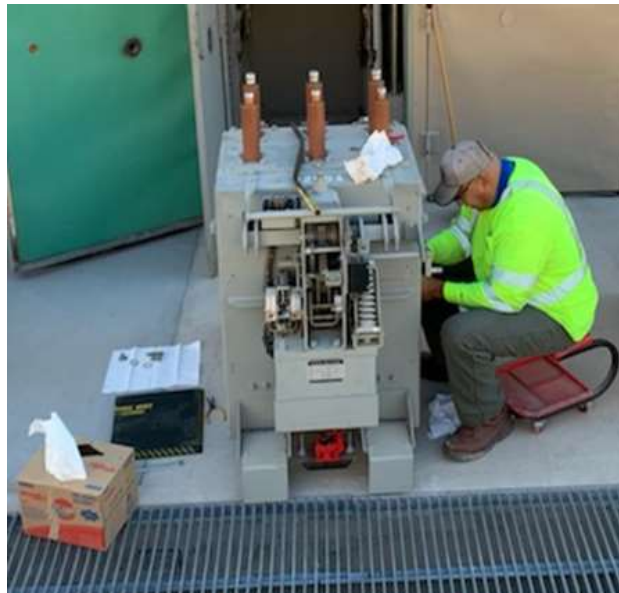
Staff performing maintenance on 6.9kV circuit breaker at Eagle Mountain pumping plant
