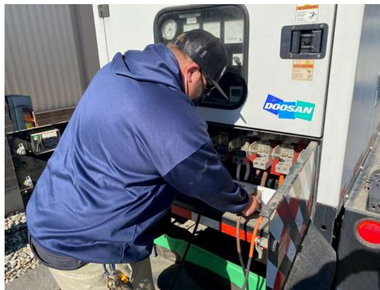
Staff connecting load bank equipment to the standby generator at San Dimas PCS
