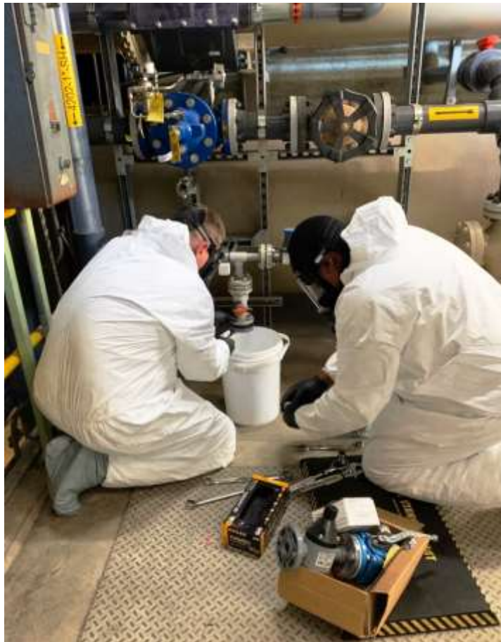
Staff changing out a valve on the sodium hypochlorite chemical system at the Weymouth plant
