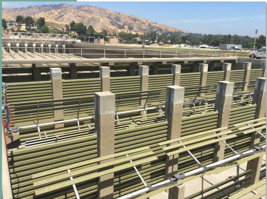
New fiberglass reinforced plastic paddle and baffle boards being installed in Basin No. 12
