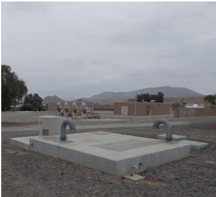
Location of tee-fitting at Lake Perris Control Facility
