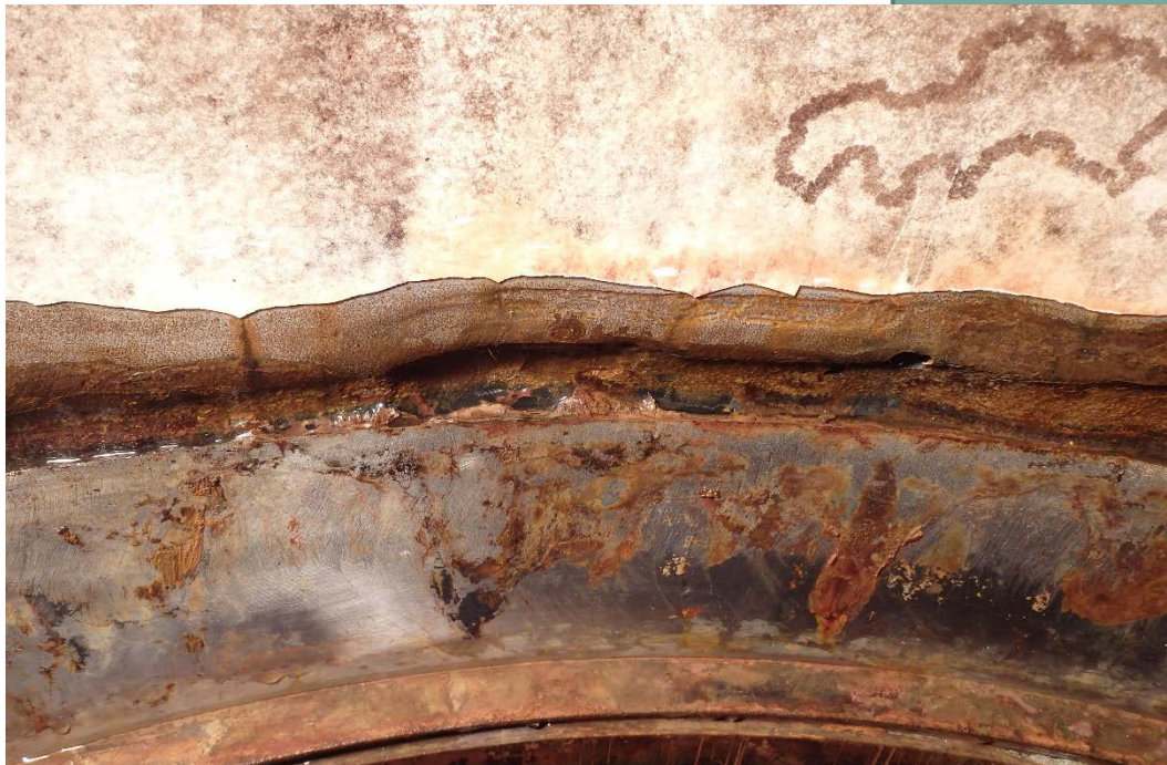
Deep pits at the stainless steel-to-carbon steel interface in Wadsworth sleeve valve Unit No. 4
