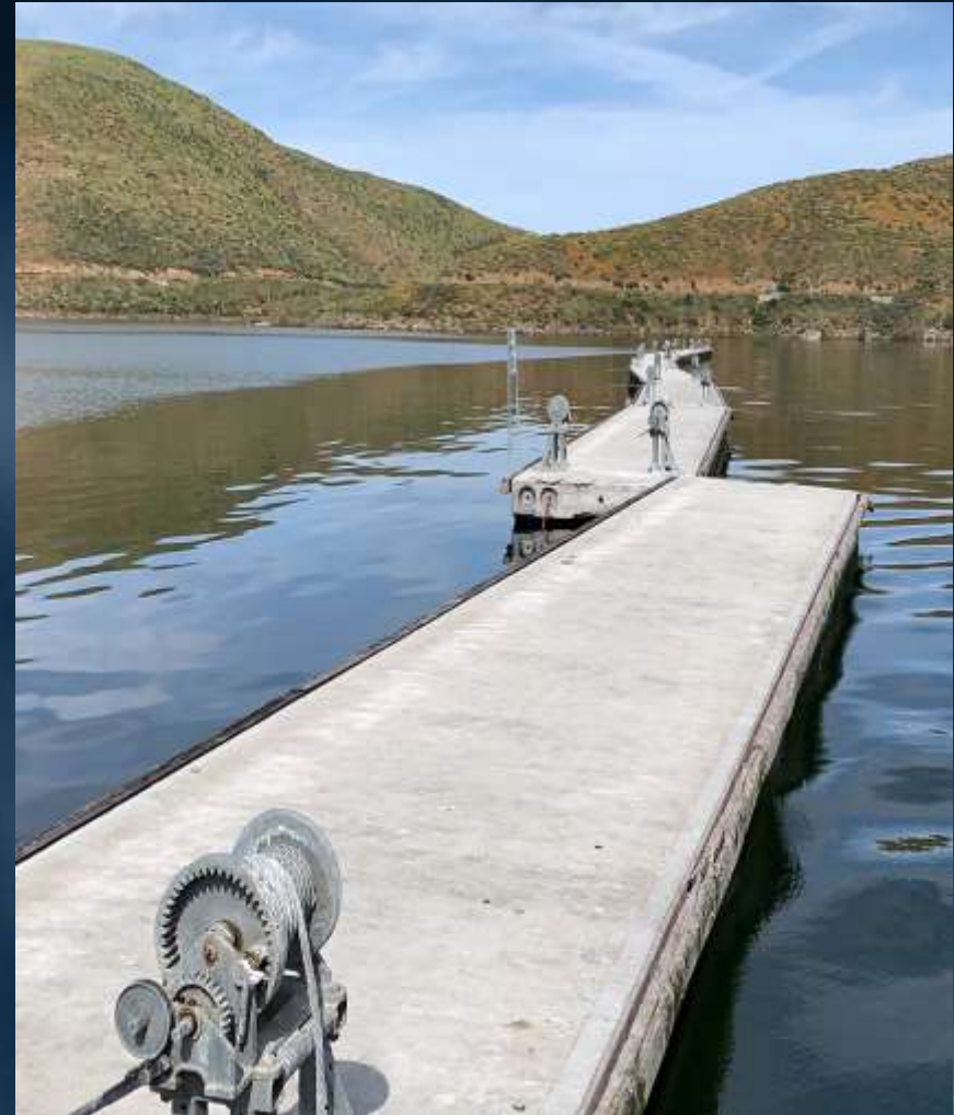
Damaged Wave Attenuator System
