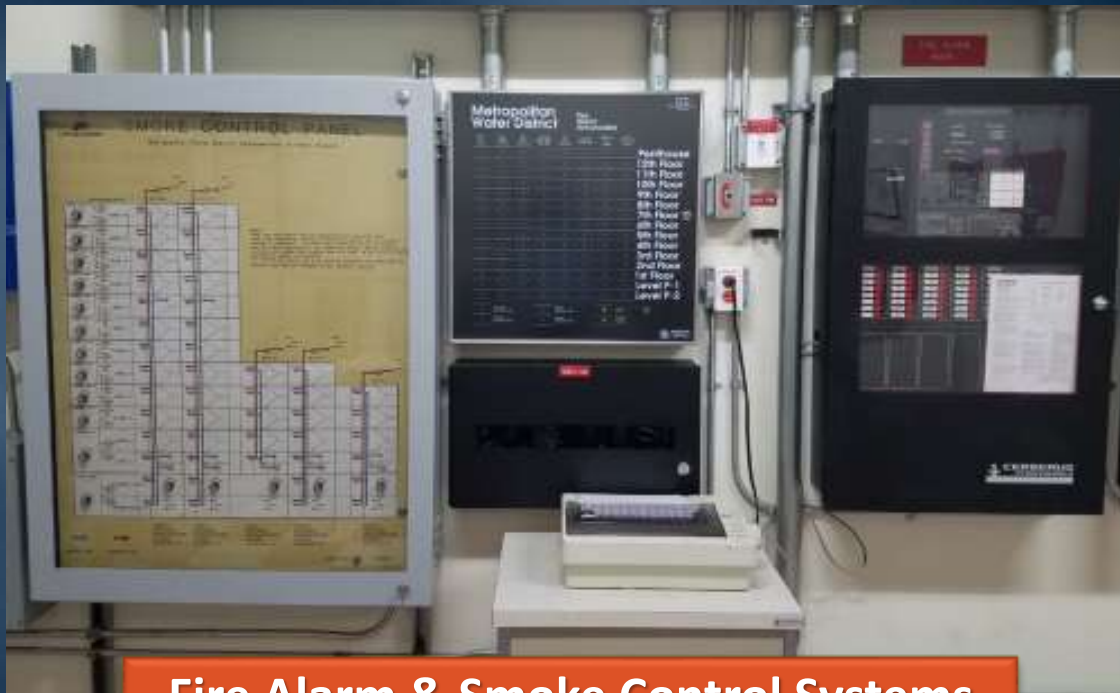
Fire Alarm & Smoke Control Systems
