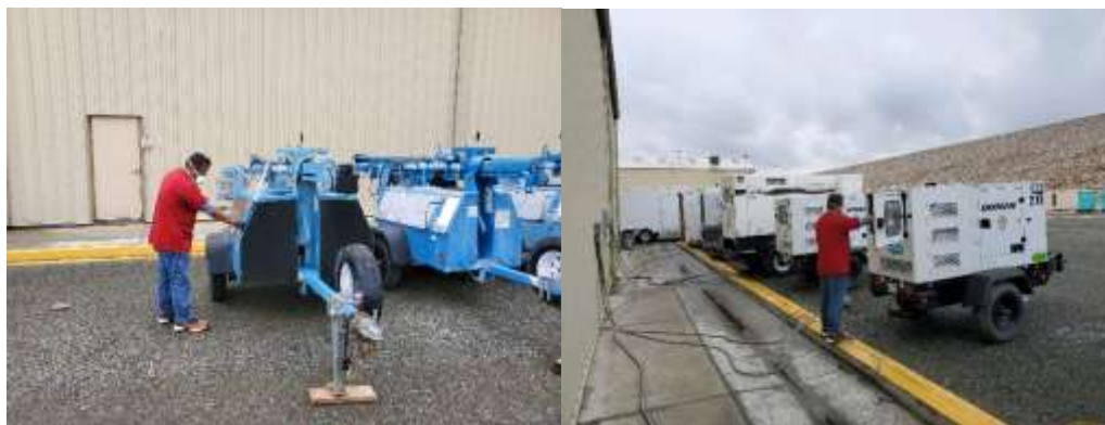
Staff performing emergency equipment checks
