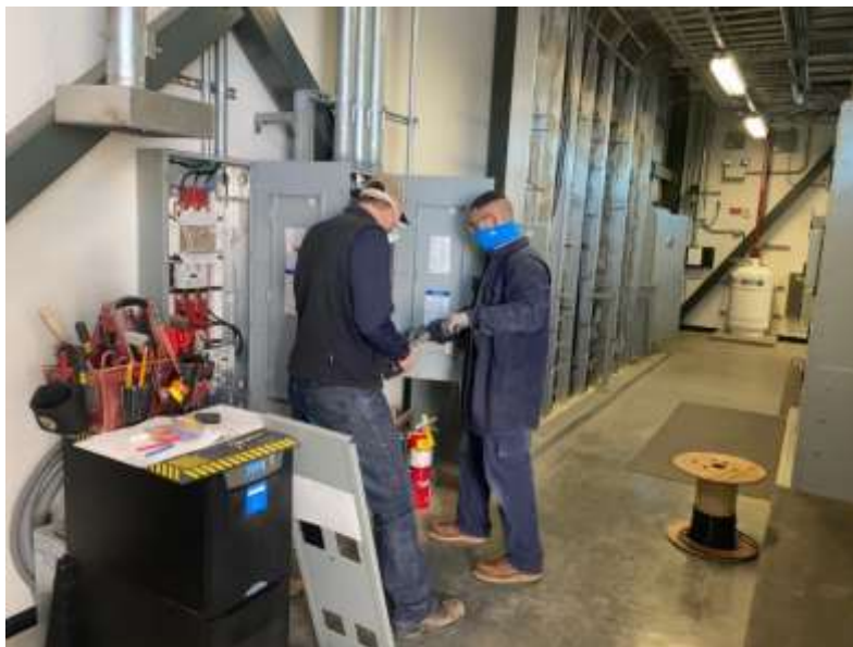
Staff replacing a UPS that is part of the ozone system at the Diemer plant
