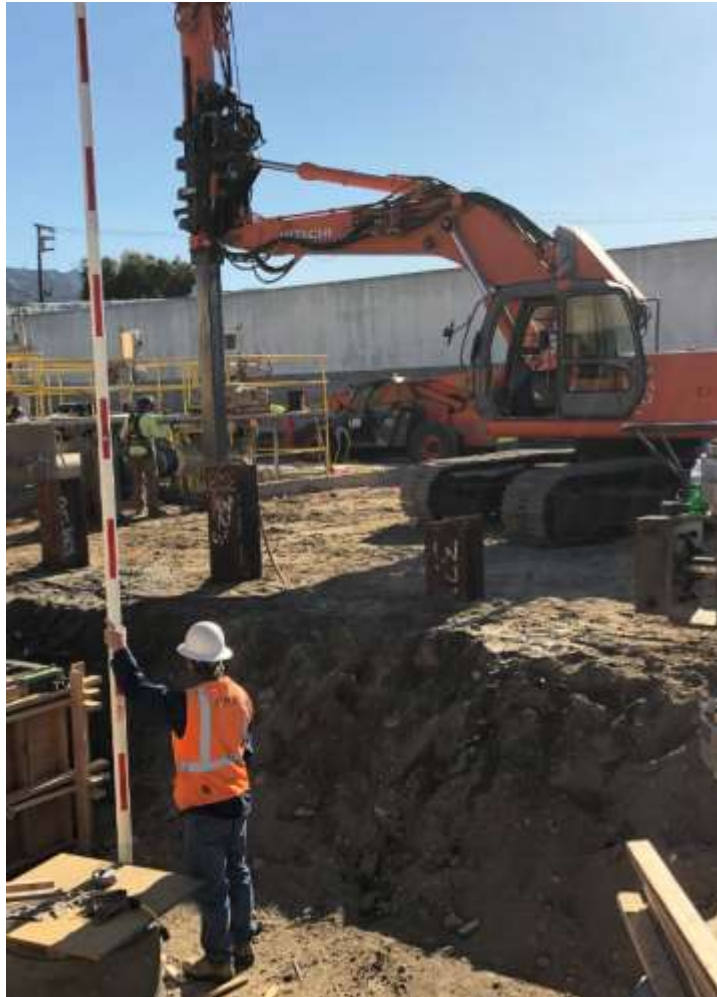
Greg Avenue Pump Station Rehabilitation – Installing shoring for the pump pad foundation
