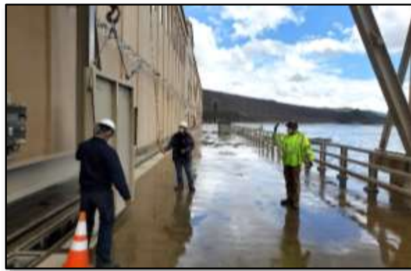
Staff removing an isolation gate at Wadsworth pumping plant while adhering to COVID-19 response protocols
