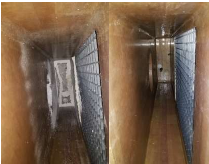
Scrubber facility before (left) and after (right) maintenance at the Jensen plant
