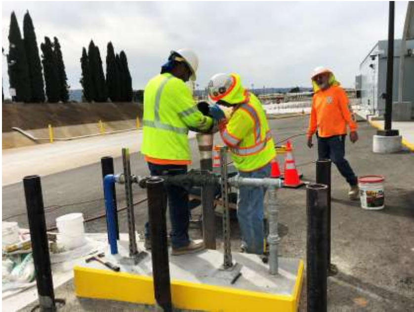
Staff installing bollards to protect a potable water line backflow preventer at the demonstration facility
