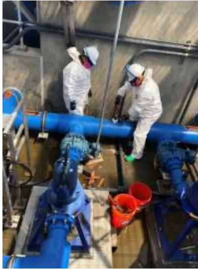
Staff modifying a return activated sludge line for the MBR system at the demonstration facility
