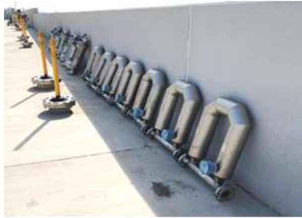
Old flow meters to be repurposed
