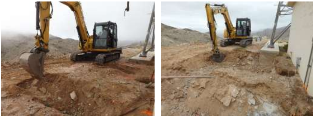
Staff excavating areas for electrical duct bank and standby generator pad for WAN project
