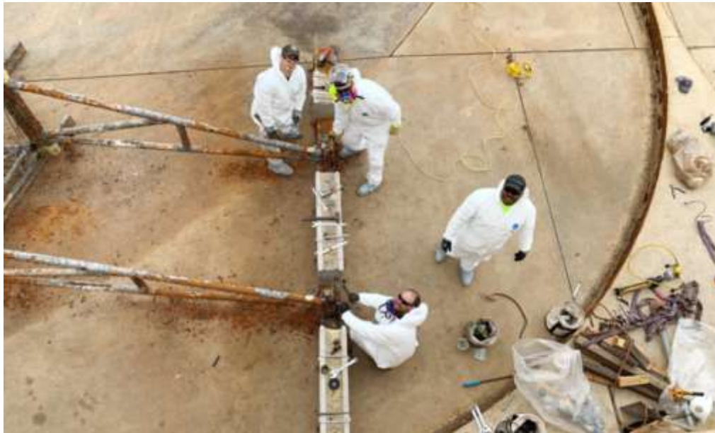
Staff removing a section of a clarifier sludge rake at the Weymouth plant.
