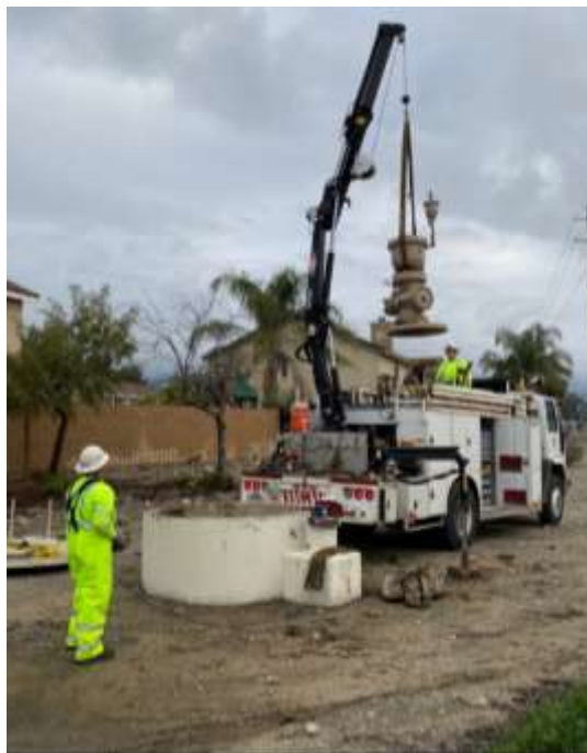
Staff removing a pipeline flange and valve assembly to access the Etiwanda Pipeline
