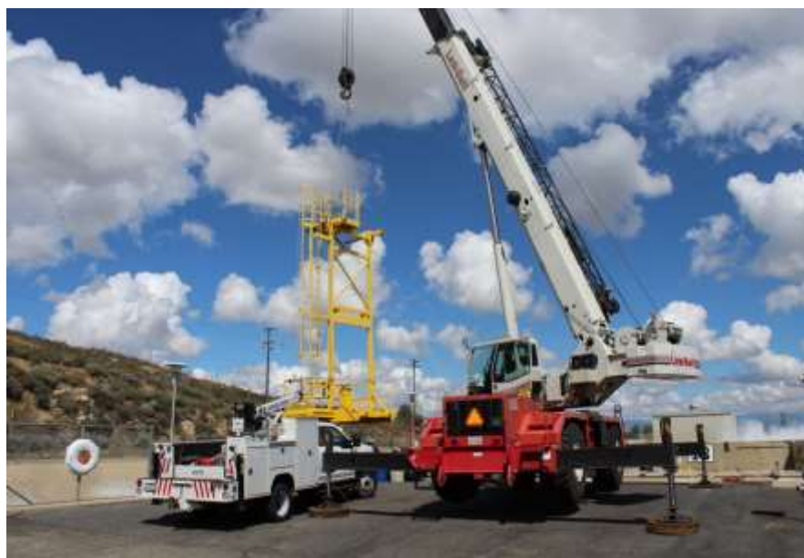
Crane hoisting the scaffolding assembly for maintaining fixed cone valves at the Lake Mathews forebay
