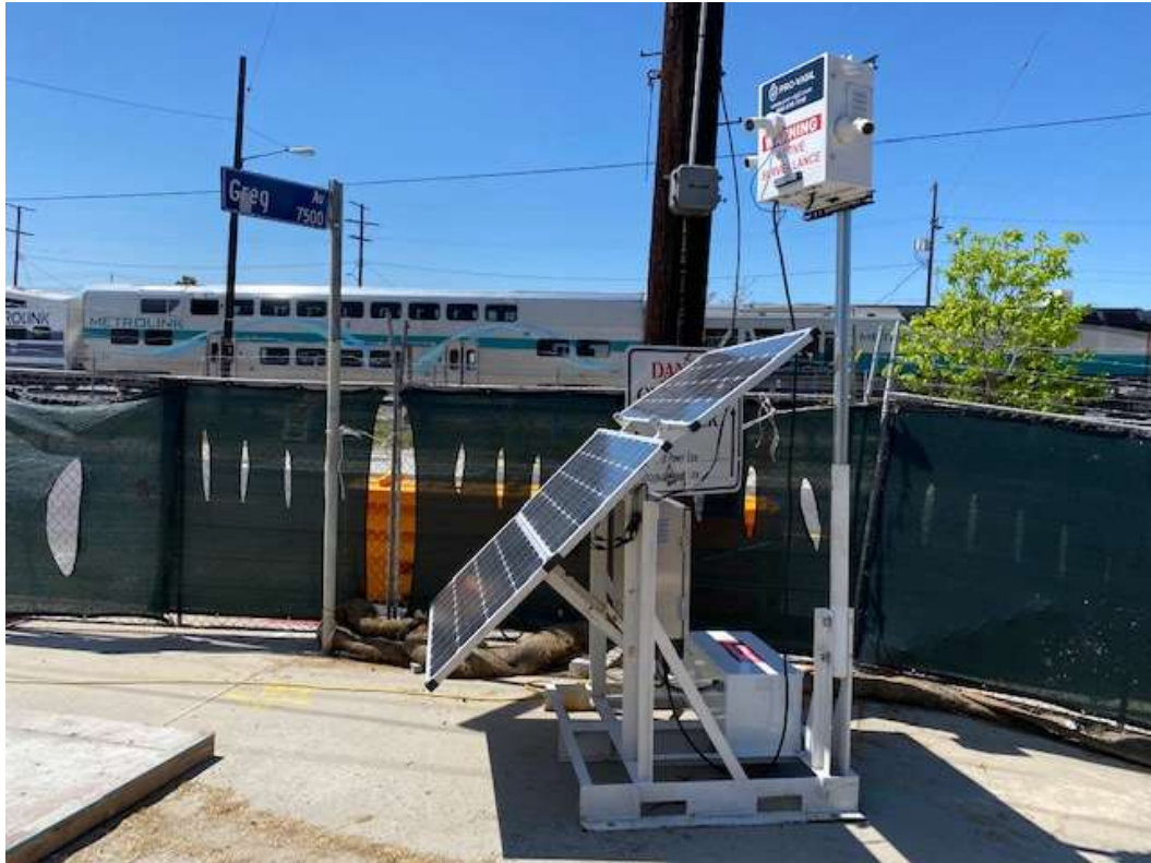
Solar panels used to power Pro-Vigil's mobile, self-sustained security surveillance device at Greg Avenue
