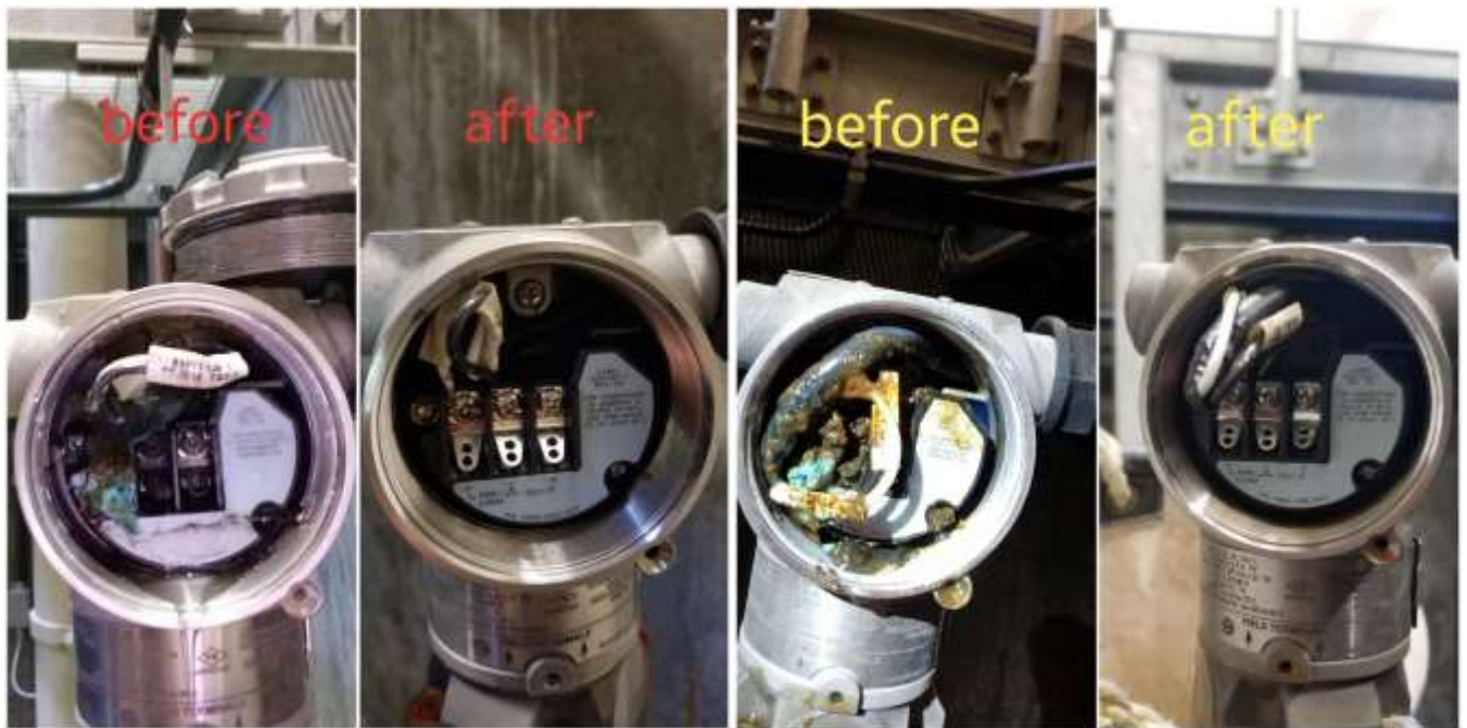
Repairs (before and after) to pressure analyzers at the CLWA-1T service connection
