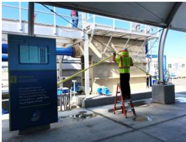
Staff installing high-visibility cable bumpers on structural cables at the demonstration facility
