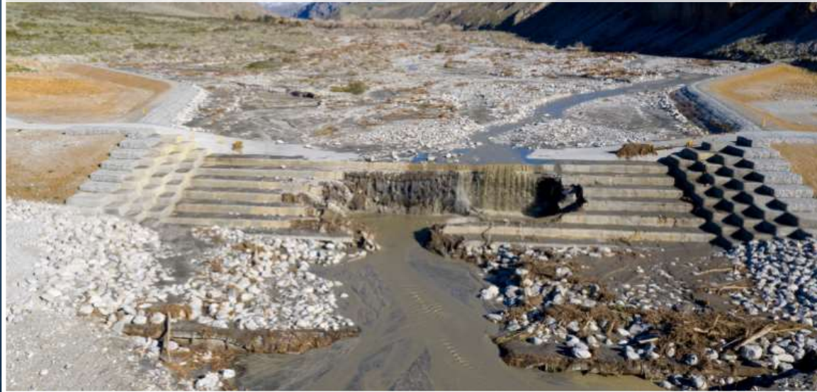
Whitewater - Damaged Erosion Protection Structure
