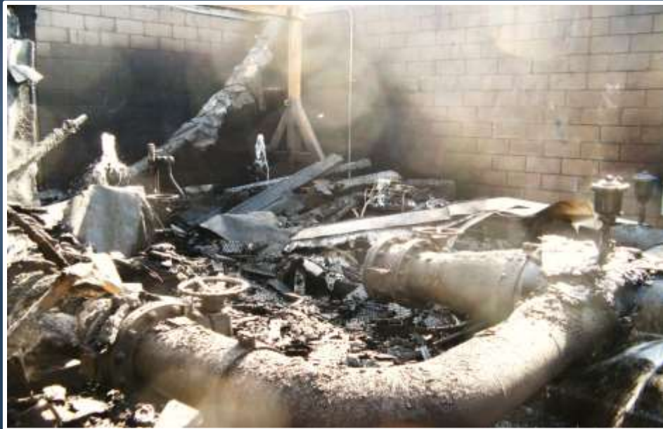
OC-71 Service Connection Structure - 2007
