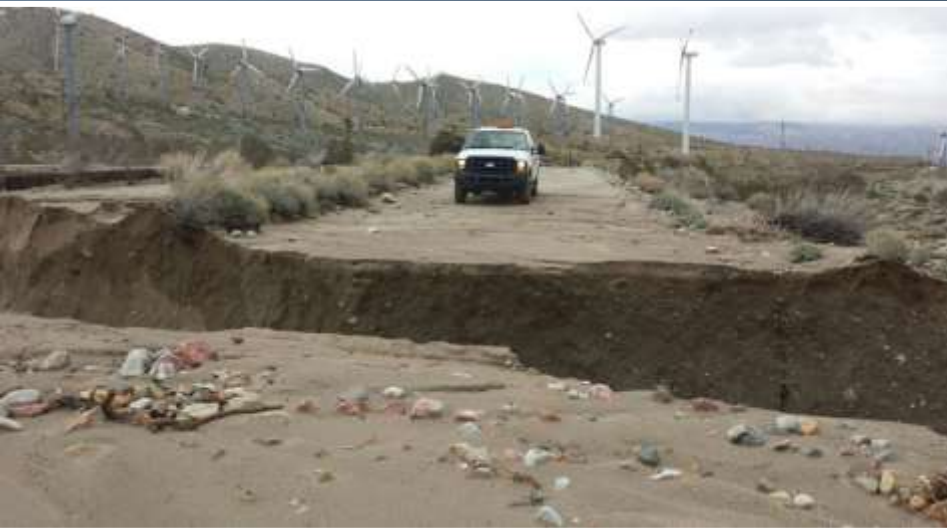
Example of Patrol Road Washout
