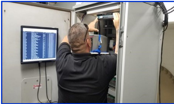
Staff performing RTU maintenance
