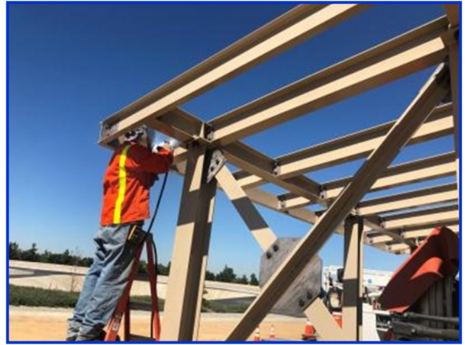
Staff welding structural steel components for a control panel canopy at the Weymouth plant
