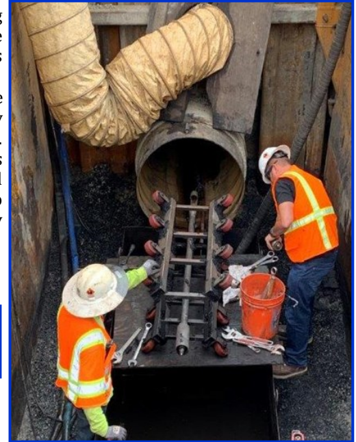
Orange County Feeder Lining Repairs – Extraction of machine that removes coal tar lining from pipeline's interior
