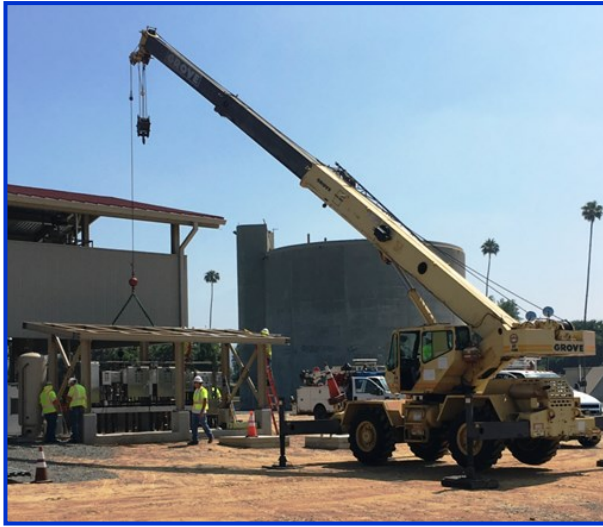
Staff utilizing a mobile crane to install a structural canopy at the Weymouth plant
