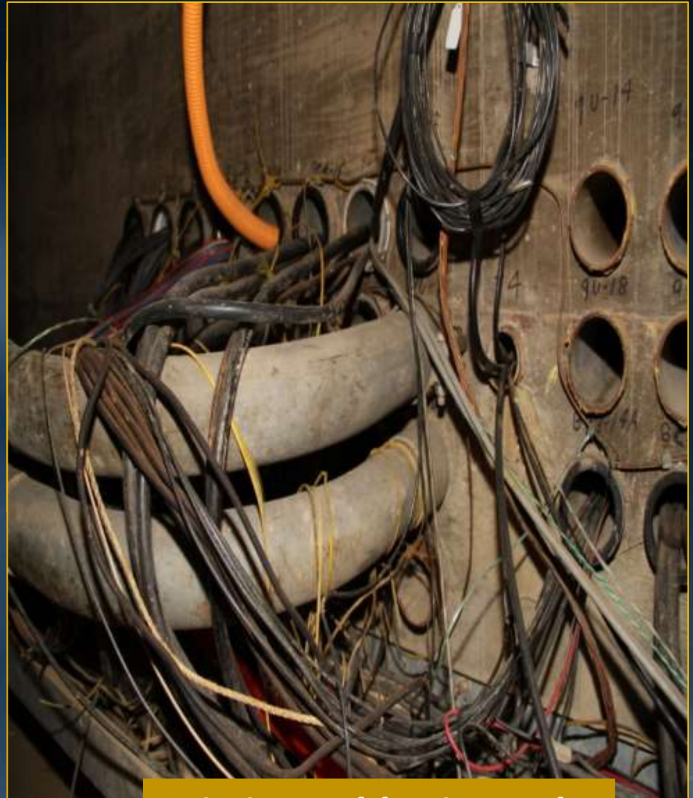
Existing Cables in Vaults
