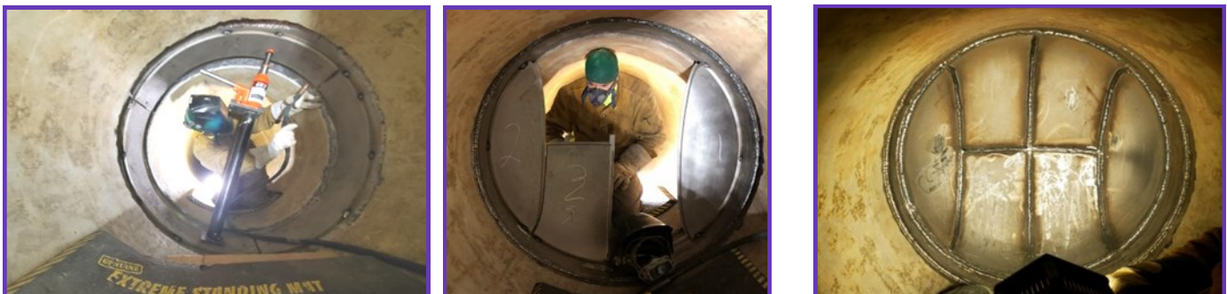
Staff welding steel band (left) and segmented bulkhead (middle), and completed bulkhead (right)
