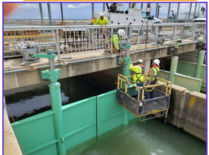
DWR installing newly manufactured wing gates at the Skinner fish control facility
