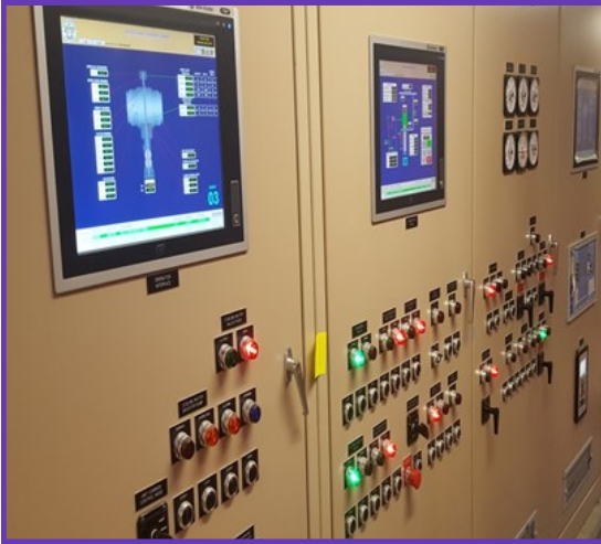
Wadsworth Pumping Plant Control and Electrical Protection Upgrade – New control systems installed
