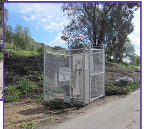
Control system equipment before (left) and after (right) security improvements
