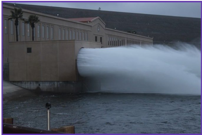
Water released into DVL forebay through fixed cone valves during pump/generator testing
