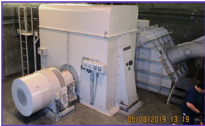
Reassembled generator at Valley View HEP
