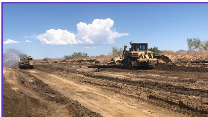
CRA Conduit Erosion Control Repairs – Grading erosion control berm adjacent to CRA
