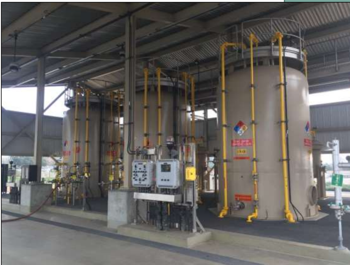
Recently upgraded Weymouth Ammonia Storage Tanks and Feed Systems
