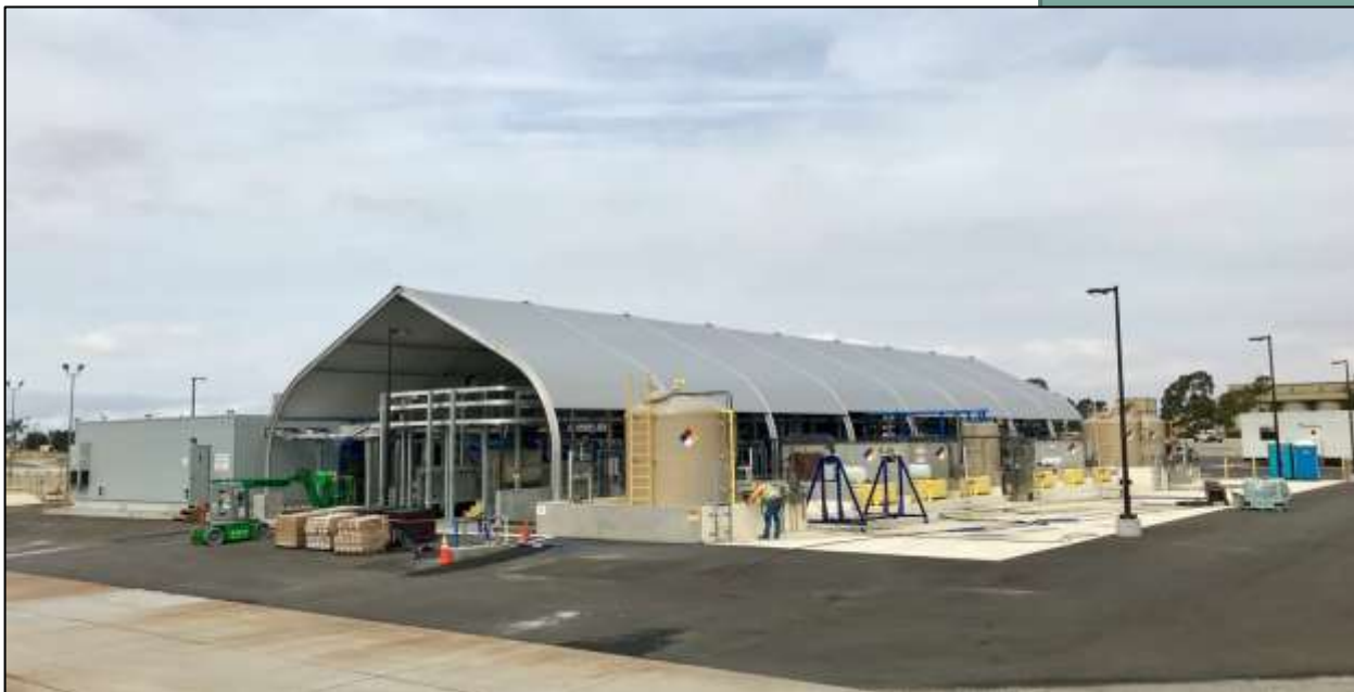
Advanced Water Treatment Demonstration Facility
