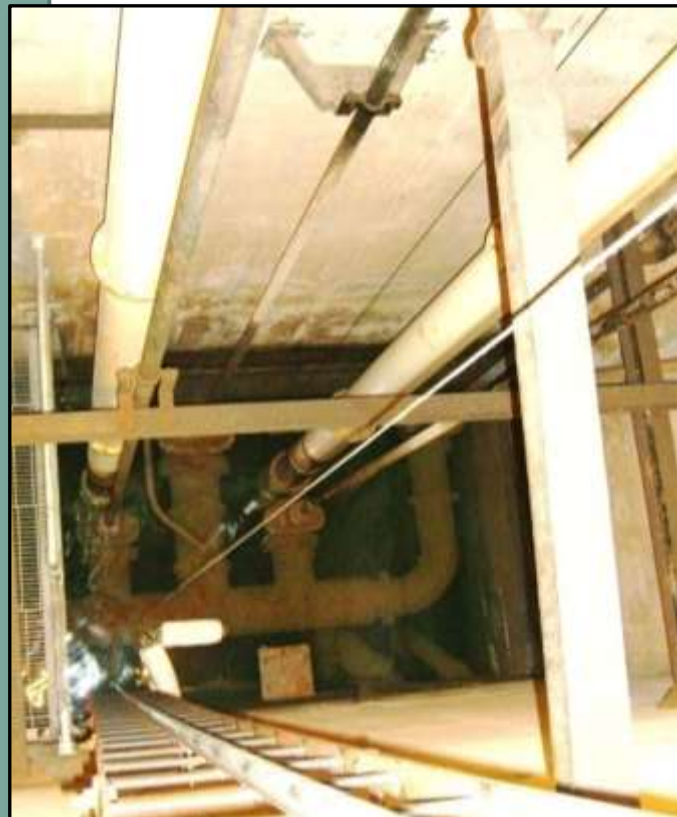
Submerged sump pumps at Iron Mountain Pumping Plant
