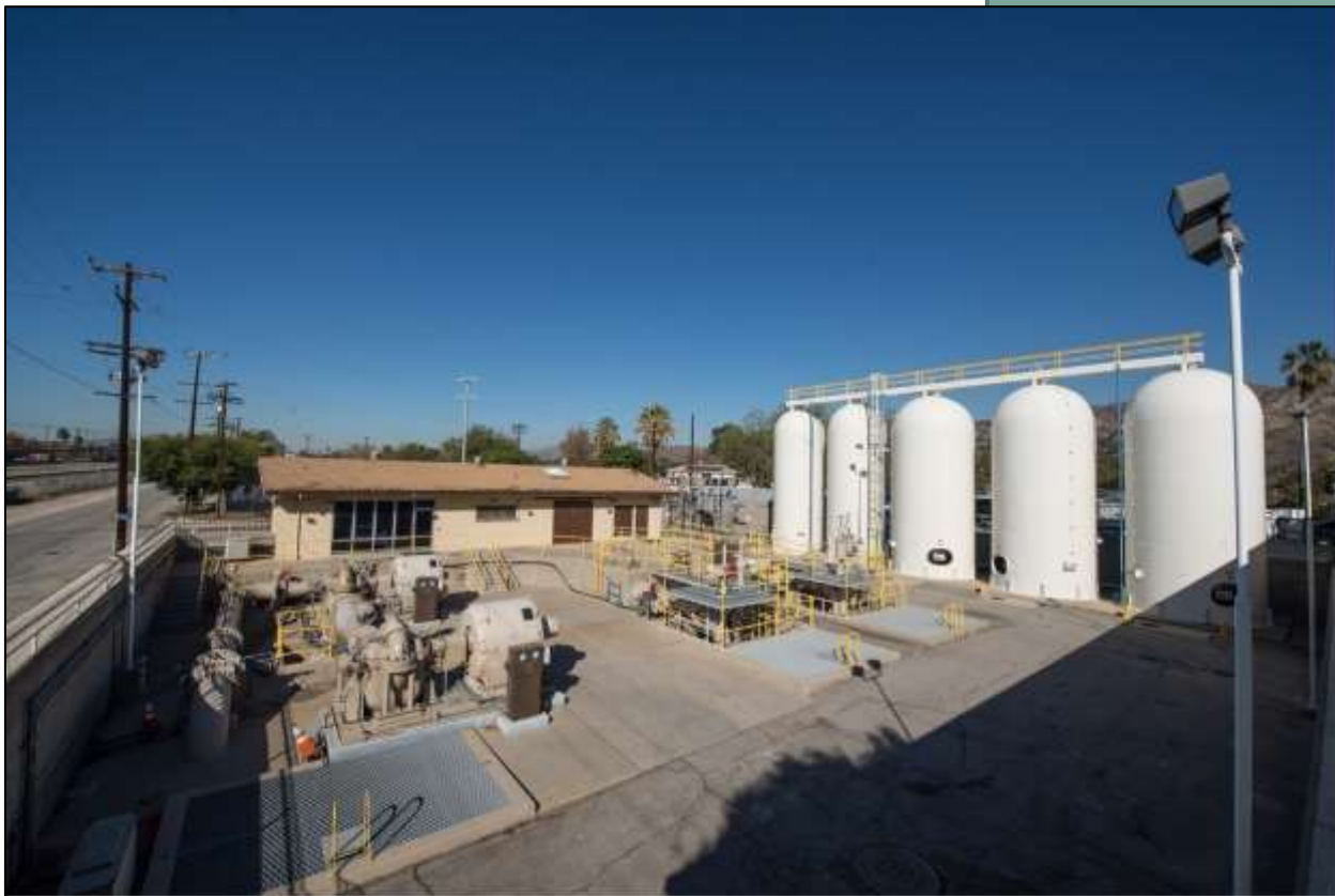
Greg Avenue Pump Station
