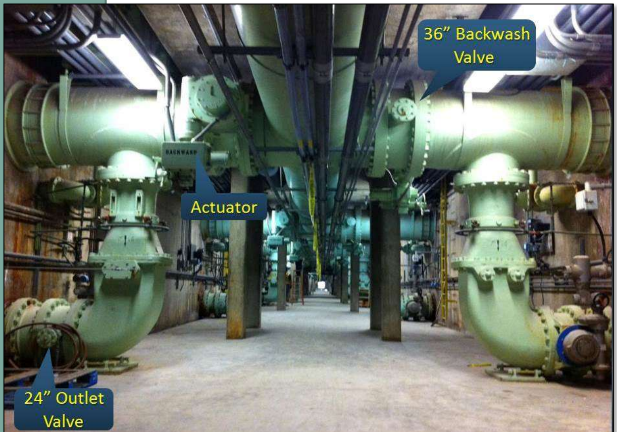
Weymouth Filter Gallery, showing equipment to be replaced
