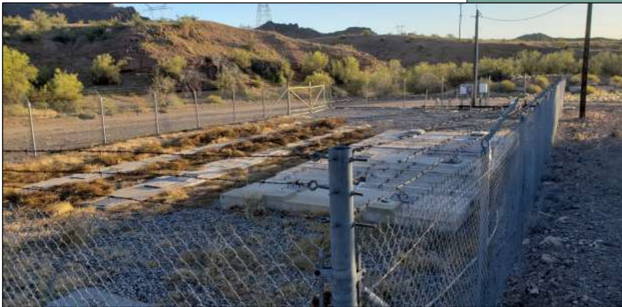
Gene Pumping Plant: septic tank/leach field
