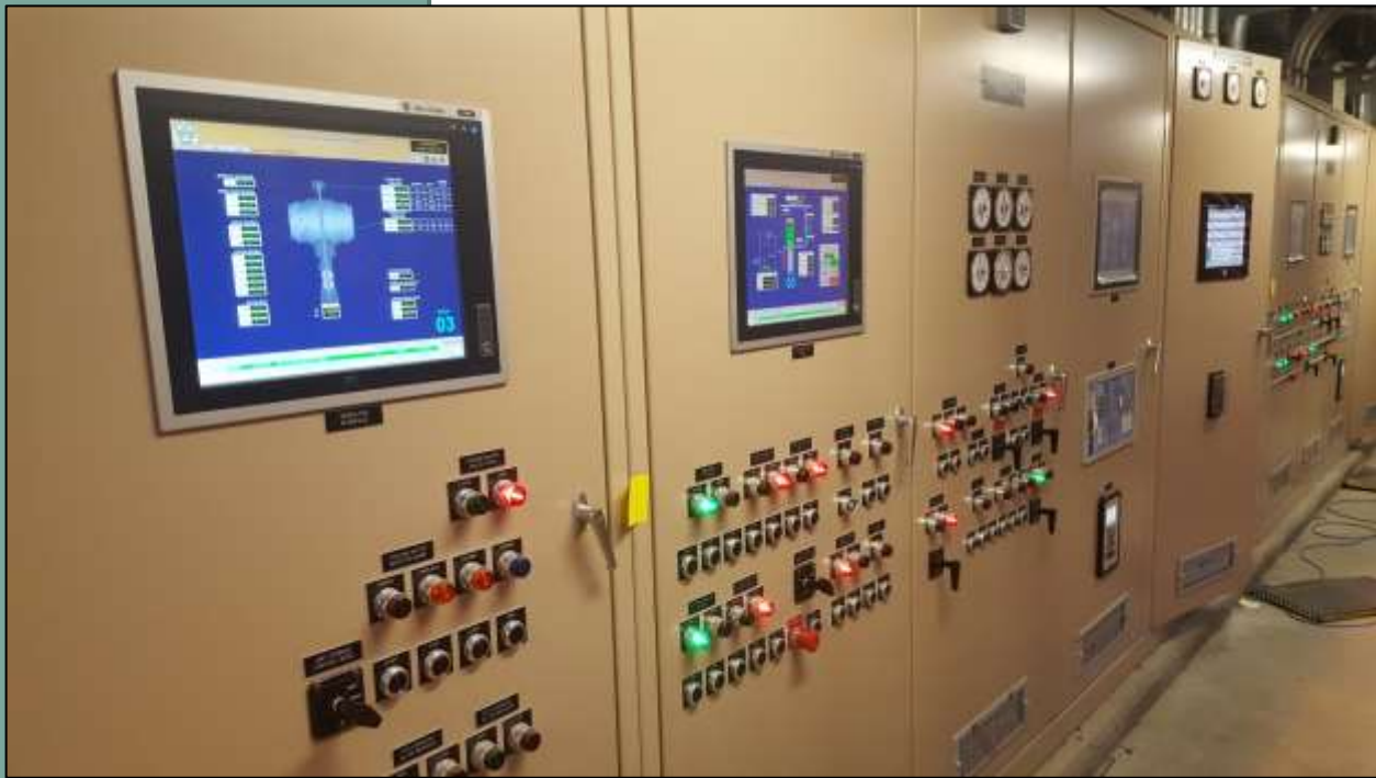
Pump/Turbine control cabinets
