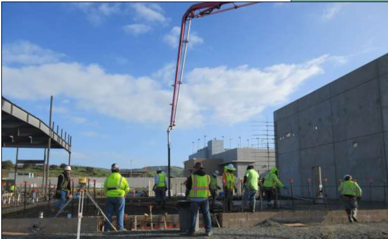
Orange County Service Center: Concrete placement at pump and valve storage room
