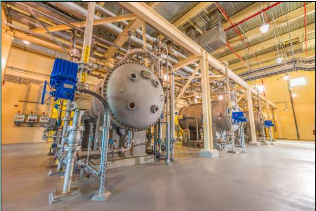
Weymouth ozone generation building
