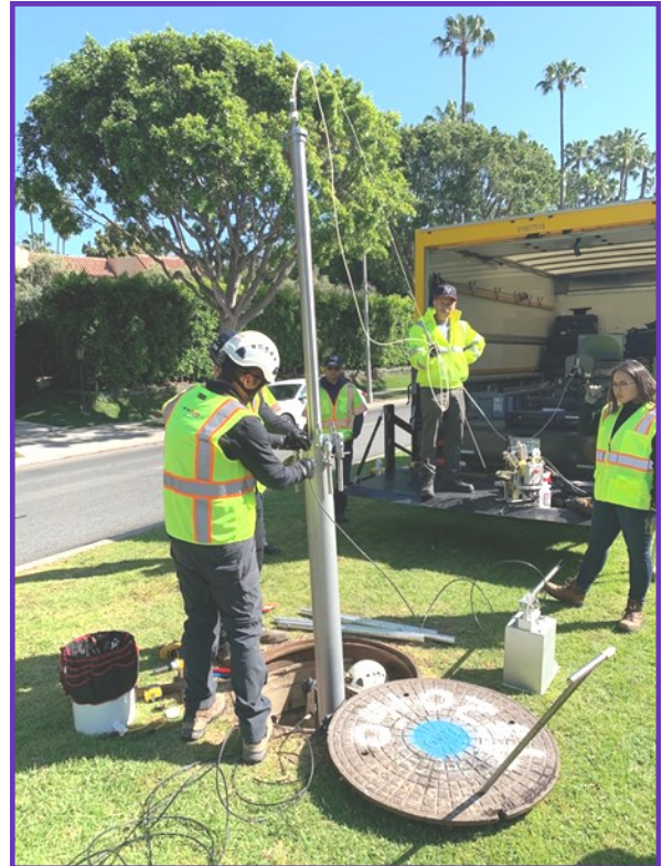
Sahara inspection tool inserted into the Santa Monica Feeder to confirm successful leak repairs
