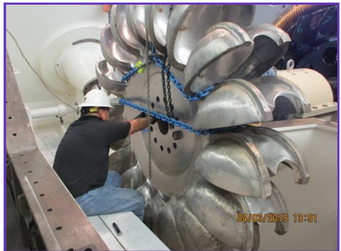
Staff securing the turbine runner to the generator shaft at the Valley View Hydroelectric Plant
