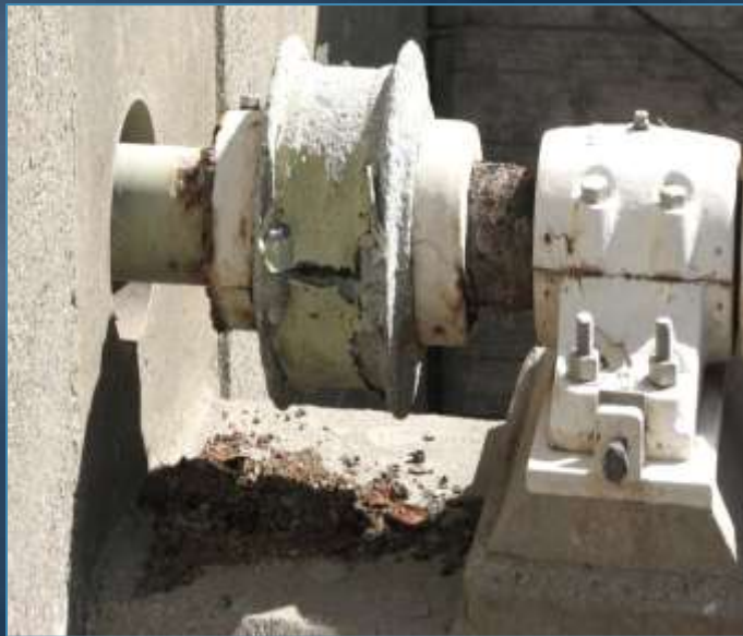
Corroded stub shafts
