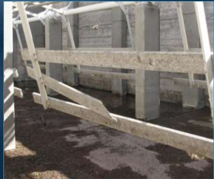
Broken baffle boards
