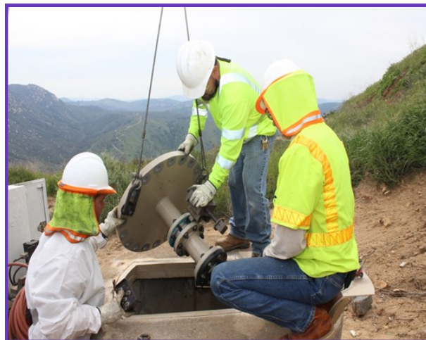
Staff removing an air release vacuum valve assembly to access San Diego Pipeline No. 2
