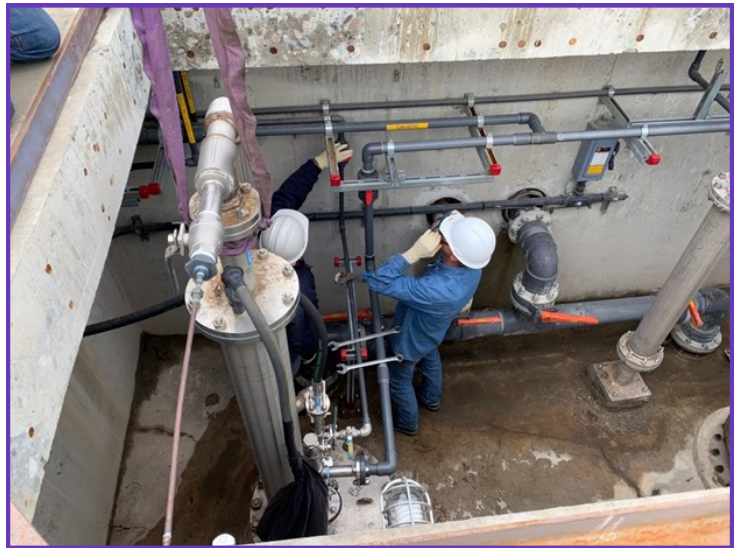
Newly installed caustic soda and ammonia mixing pump in the CFE channel at the Jensen plant
