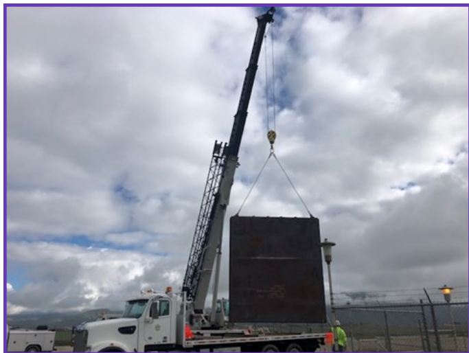
Staff installing a newly manufactured drop gate along the Casa Loma Canal
