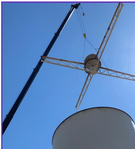
F.E. Weymouth Water Treatment Plant, West Washwater Tank Seismic Upgrades – Removal of center roof support and Removal of center roof support
