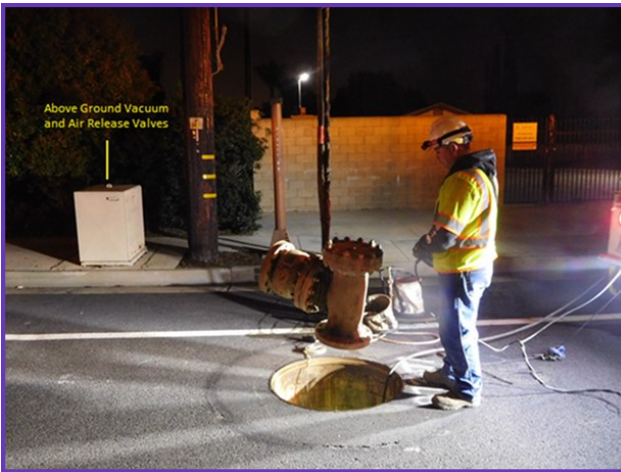
Staff removing flanges and equipment to support PCCP relining of the Second Lower Feeder
