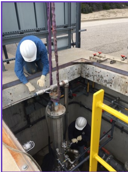
Staff removing the caustic soda and ammonia mixing pump at the Jensen plant
