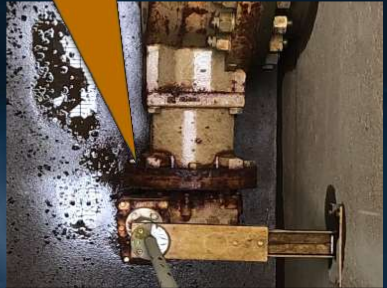
Inlet Valve Gearbox
