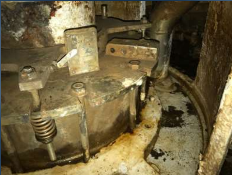
Corroded mechanical seal & turbine shaft
