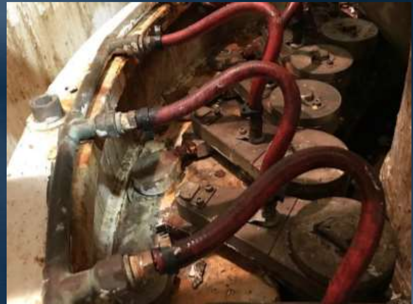
Corrosion on wicket gate operator
