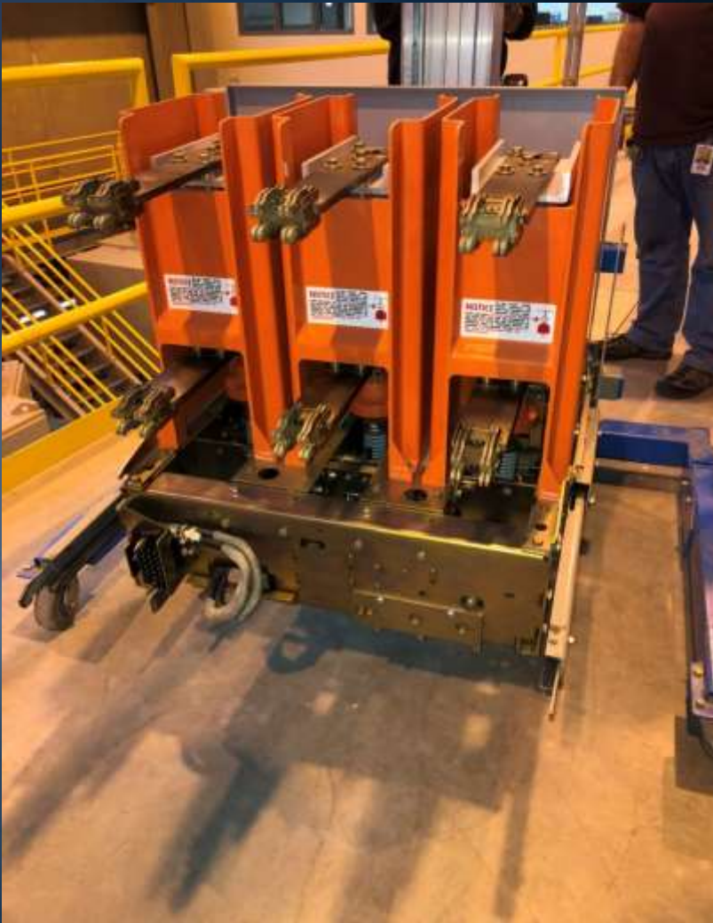
Back side of circuit breaker
