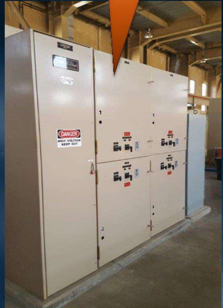
Circuit breaker cabinets
