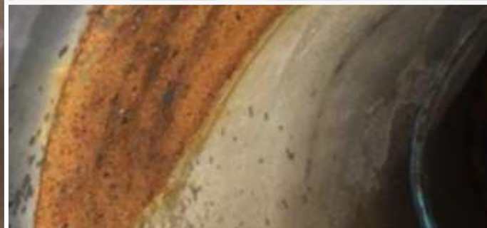
Mortar Lining Damage
