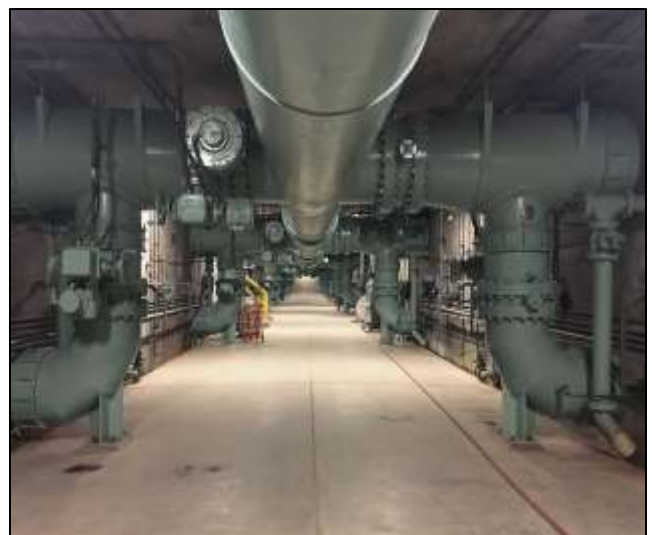
Diemer Plant New backwash and filter outlet valves in filter gallery
