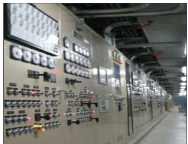
Wadsworth Pumping Plant Pump/turbine control panels
