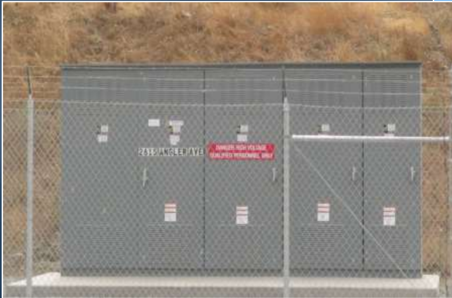
Electrical switchboard at Marina
