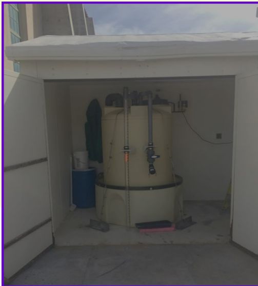
The new sodium hypochlorite tank at Eagle Mountain pumping plant.
