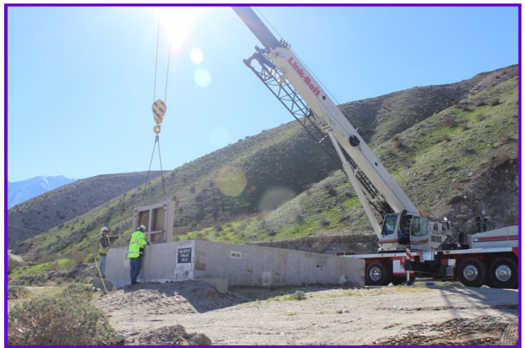
Installation of a flow blocking gate at the Whitewater Siphon on the Colorado River Aqueduct.
