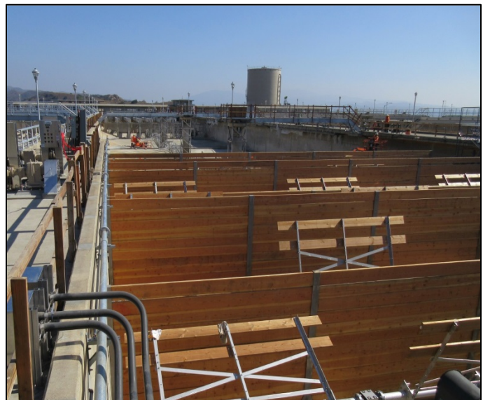
Diemer Plant Flocculation basins
