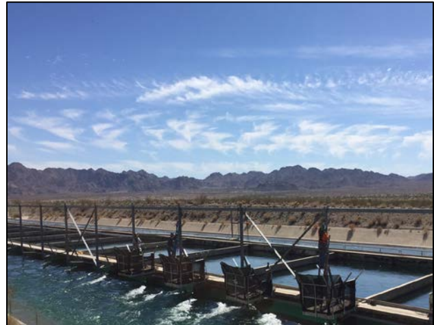
CRA Sand Trap Structural steel support for electrical conductors near Hinds Pumping Plant
