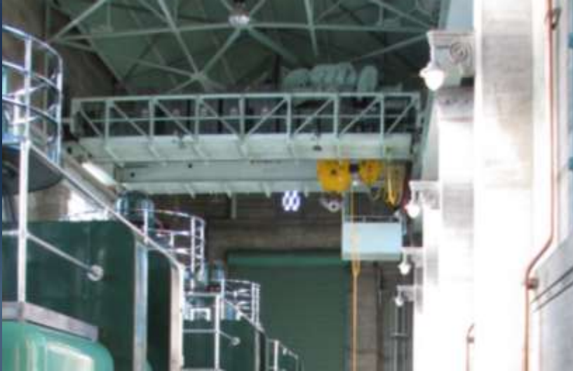
CRA Pump House Bridge Cranes
