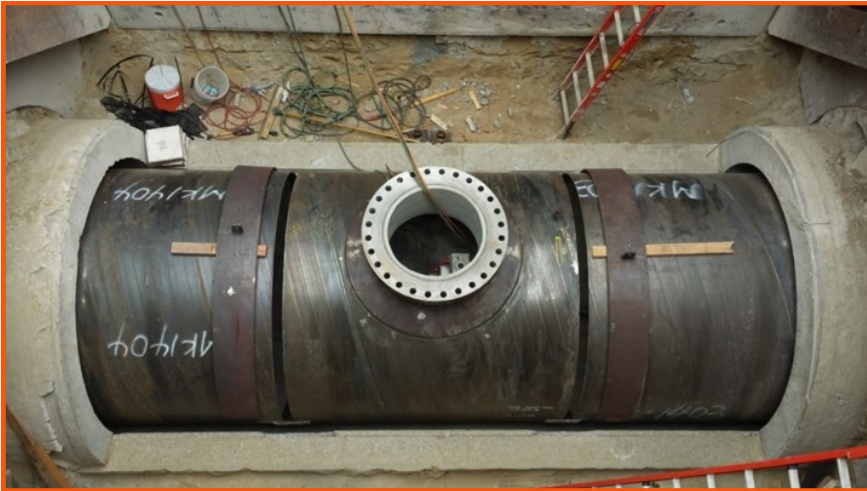
Completion of the new pipe segments at a construction entrance site on Haynes Street in Los Angeles.
