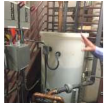
Tank collects distillate water which is then pumped to the main co-generation plant
