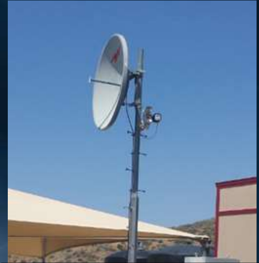
East Marina WAN tower
