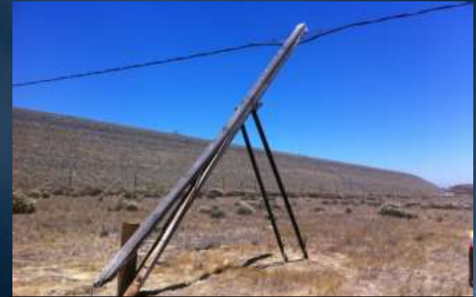
Damaged temp. power pole
