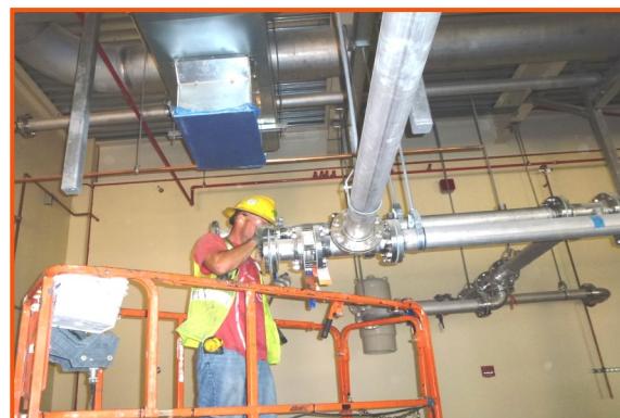
Weymouth-Piping within chiller room
