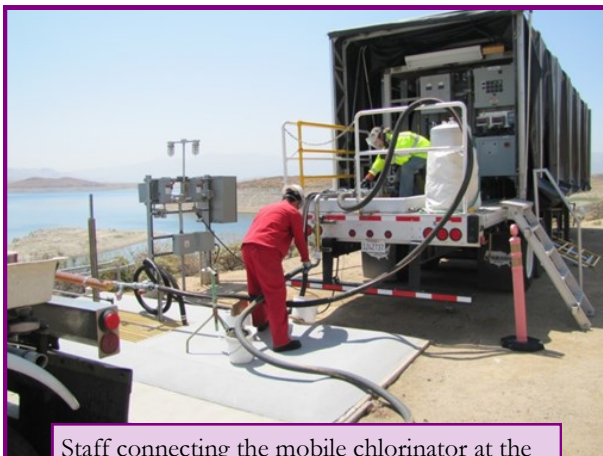
Staff connecting the mobile chlorinator at the Lake Mathews Outlet Tower
