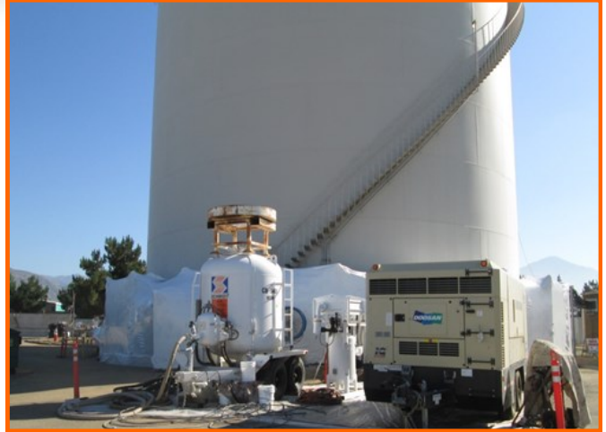
Weymouth East Washwater Tank Seismic Upgrades—Preparations for sandblasting and coating of new tank anchorage system.
