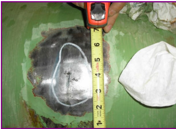
Service Connection FM-1 venturi meter pinhole leak on the Upper Feeder
