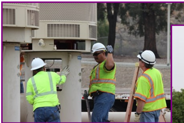
Staff reinstalling electric motor (left) and pump shaft and electrical connections (right) at the Perris Pumpback facility.
