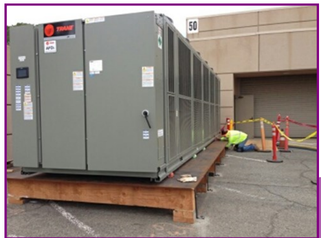
The new chiller unit installed on a temporary platform for the Water Quality Laboratory
