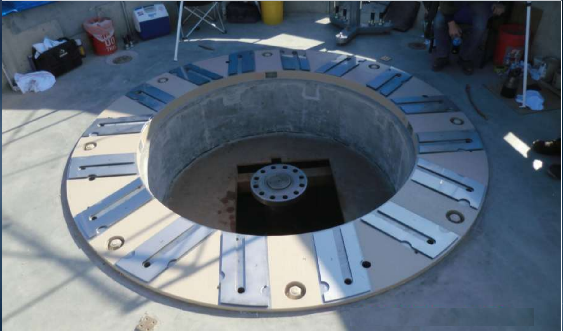
Sole Plate - machined, faced, painted and shimmed
