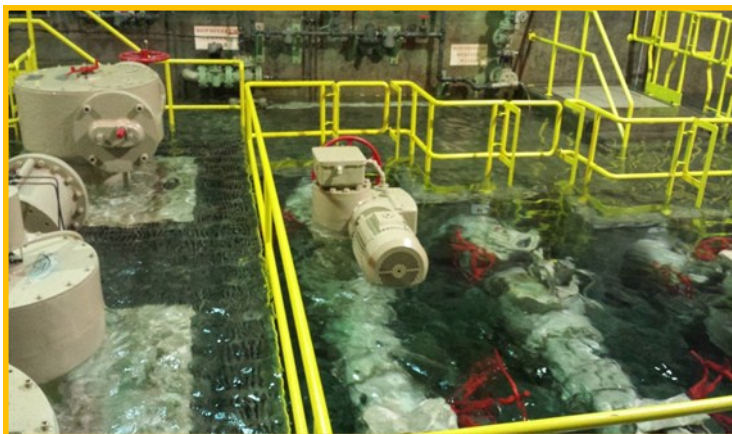
Inundation of the San Gabriel PCS on the Lower Feeder
