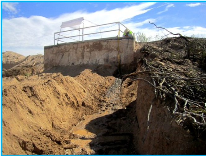
Excavation of the Siphon Transition Structure to expose the seepage point along the CRA
