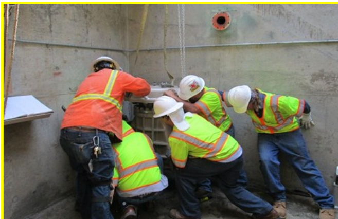
Staff installing the newly refurbished 16-inch control valve in the Hollywood Control Structure on the Santa Monica Feeder
