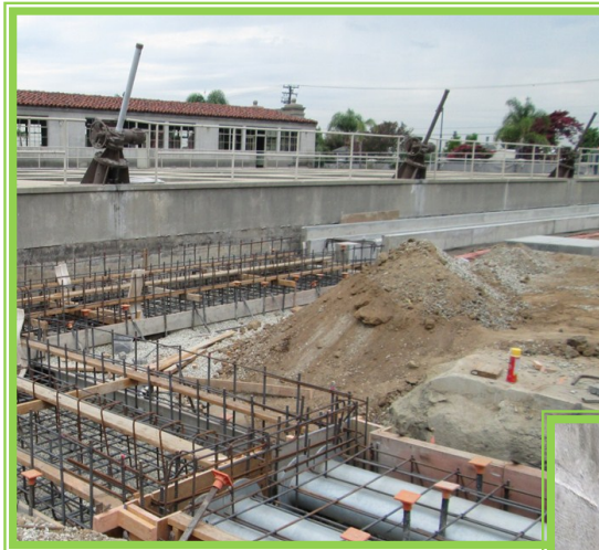
Weymouth Filter Outlet Chemical Trench—Pipe encasement for the sodium hydroxide and ammonia lines at a road crossing
