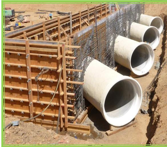
Weymouth ORP—Plant overflow discharge structure
