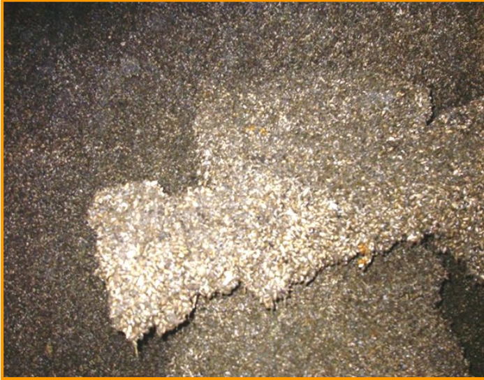
Before cleaning: Dense layer of quagga mussels attached to a Tier No. 4 valve (above normally operated chlorine injection point)
