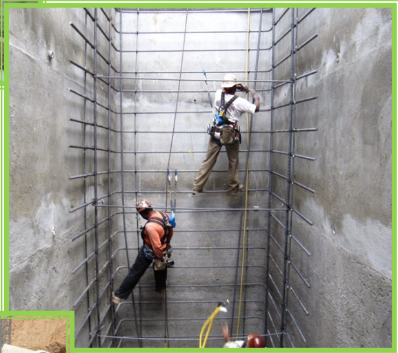
Diemer Finished Water Reservoir and East Washwater Tank Seismic Upgrades—Installation of reinforcing steel within the south shear wall of the reservoir
