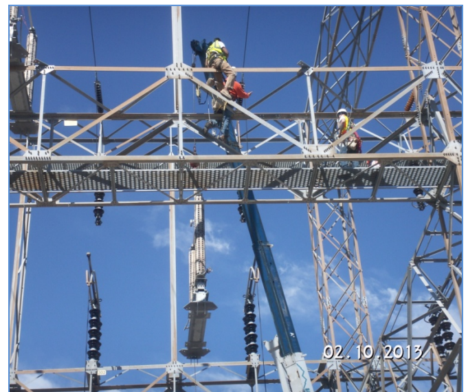
CRA Pumping Plants High voltage disconnect switch
