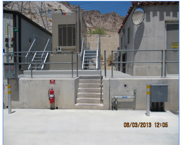
Hinds Pumping Plant New standby generator
