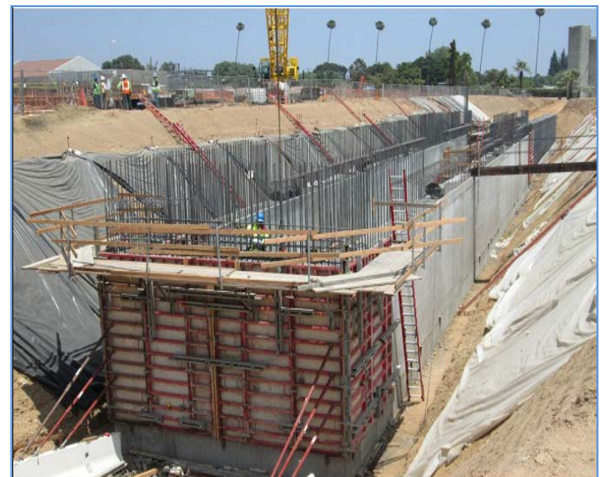
Weymouth Plant Ozone Contactor Inlet Conduit
