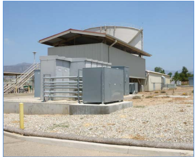
Weymouth Plant New electrical substation
