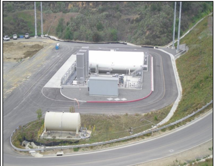
Diemer Plant Liquid oxygen (LOX) tank farm
