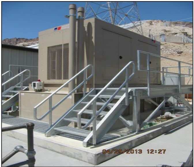
Hinds Pumping Plant New standby generator
