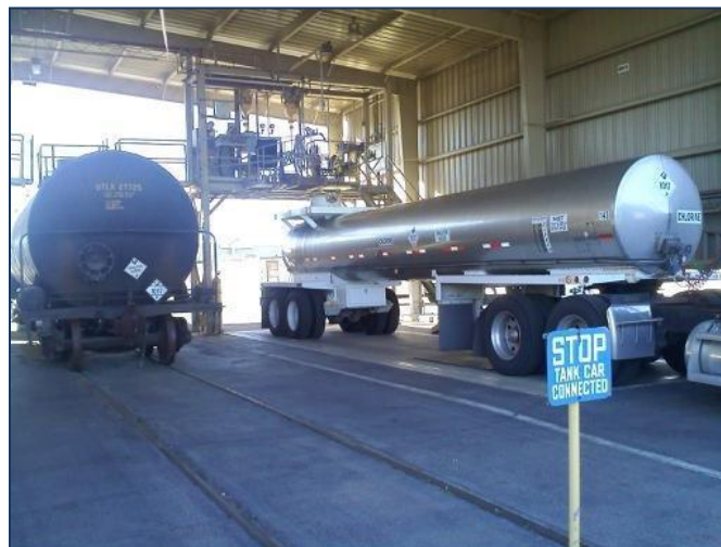
Existing Chemical Unloading Facility
