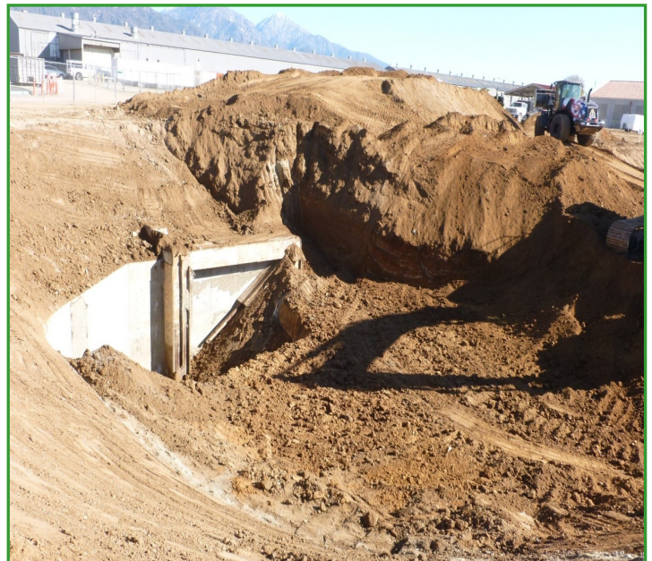
Weymouth ORP – Connection Point for Ozone Contactor Inlet Conduit
