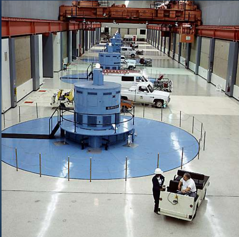
Inside Hyatt Power Plant
