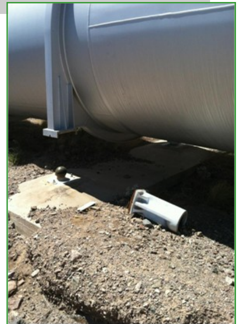
Broken support assembly at pump plant delivery line at Gene
