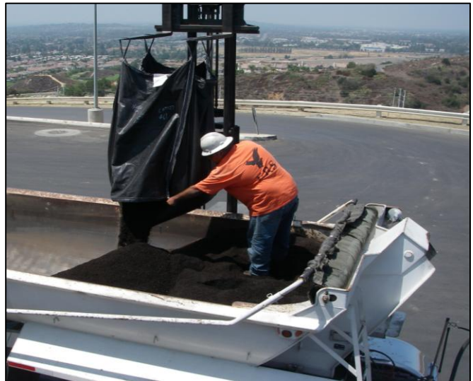
Diemer Plant Filter media replacement
