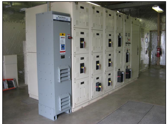
Skinner Plant High-resistant ground fault equipment installed in Electrical Building No. 3
