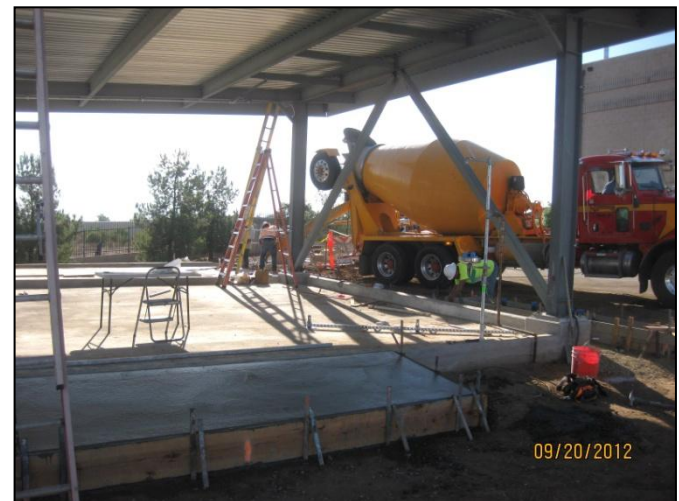
Mills Plant Placement of concrete for the Hazardous Waste Staging and Containment Facility
