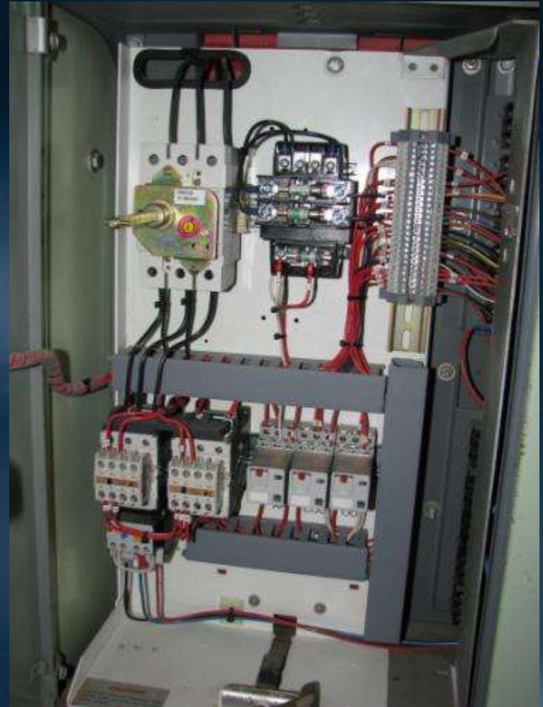
Upgraded MCC Bucket
