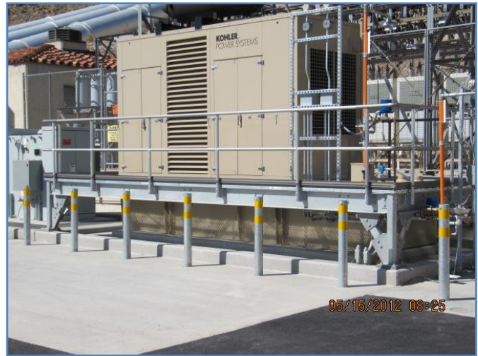
Eagle Mountain Pumping Plant New standby generator
