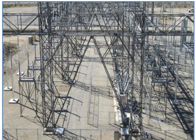
Colorado River Aqueduct High voltage disconnect switches
