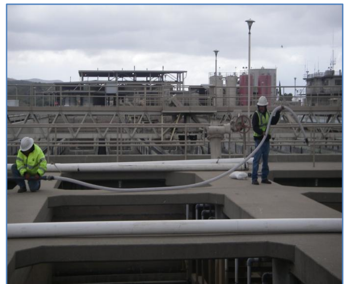
Diemer Plant Filter bays
