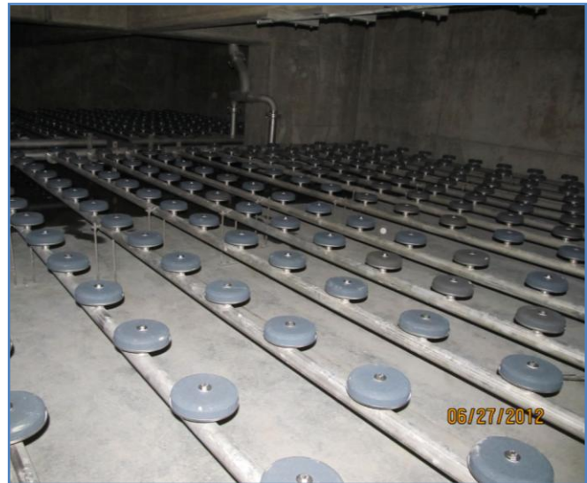
Diemer Plant New ozone diffusers
