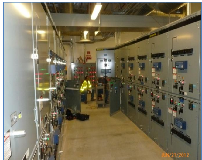
Weymouth Plant New ORP switchgear
