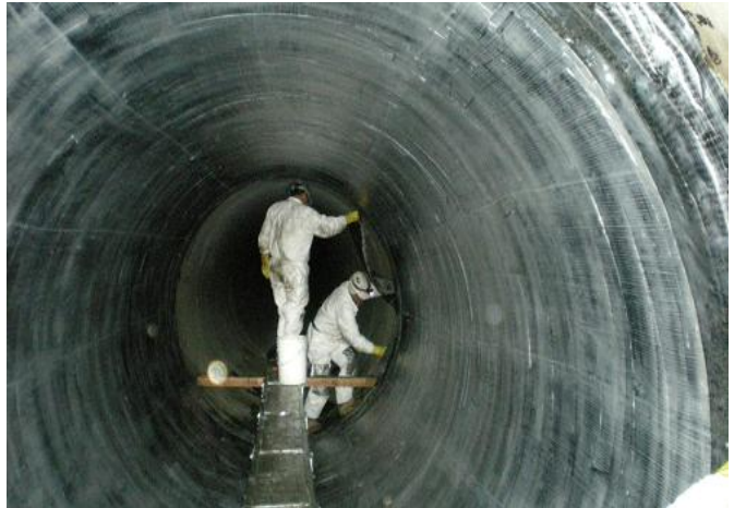
Carbon fiber-wrapped pipe segment Sepulveda Feeder
