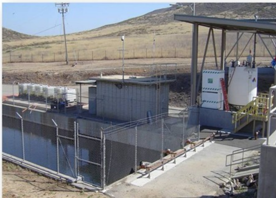
The new sodium bisulfate facility in operation at the inlet of Lake Skinner
