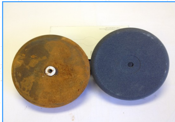
Degraded (left) and replacement (right) diffusers at the Jensen water treatment plant.
