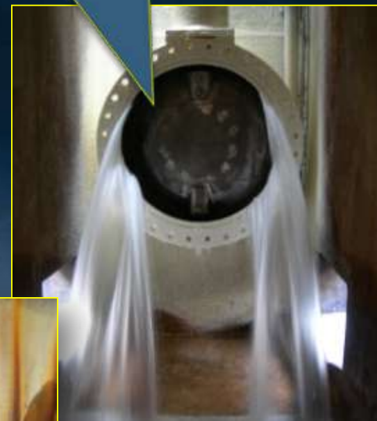
Leaking valve with disk closed
