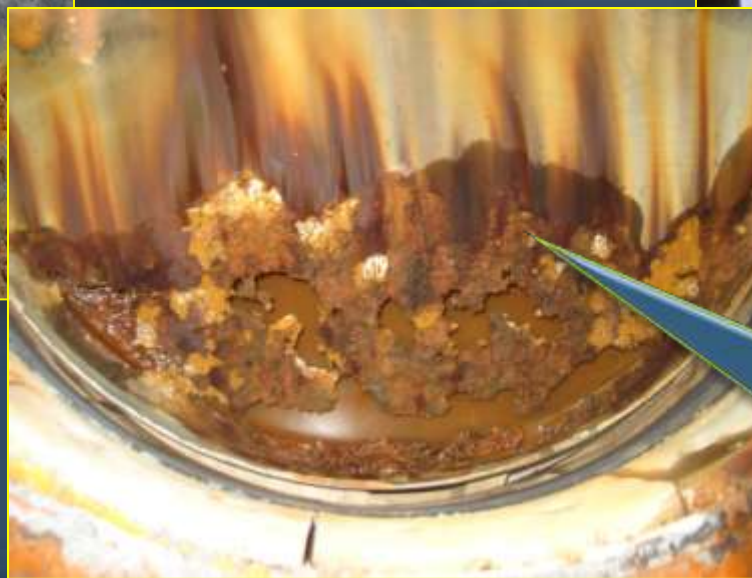
Corroded valve disk with failed coating & metal wastage
