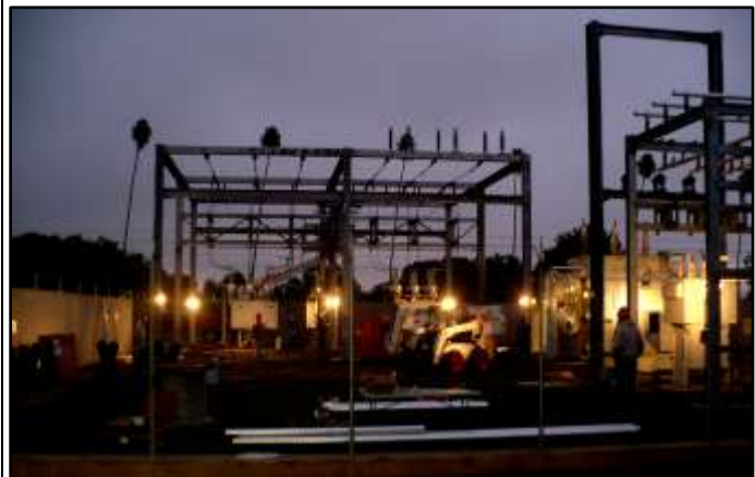
Weymouth Plant New Electrical Switchyard
