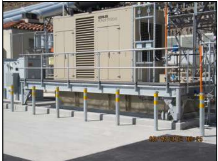
Eagle Mountain Pumping Plant New Standby Generator
