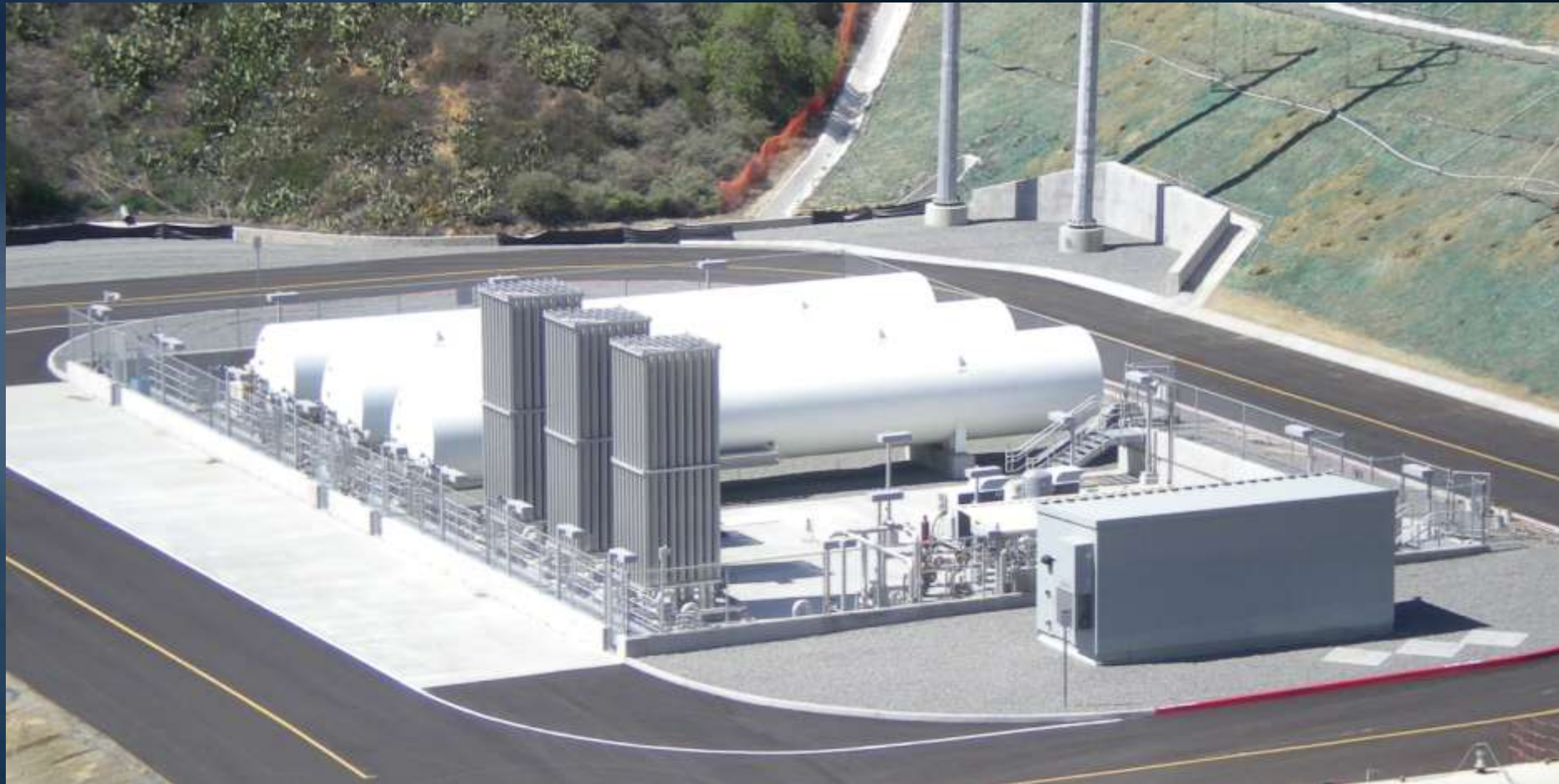
Liquid Oxygen Storage Tanks
