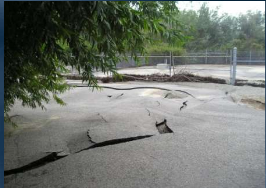
Olinda Pressure Control Structure
