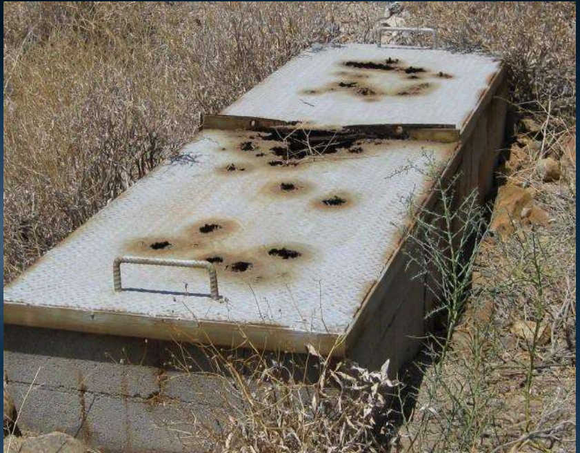
Distribution Box at Hinds P.P.
