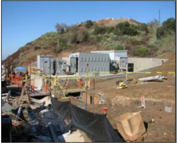
Diemer Fire and Potable Water Pump Station
